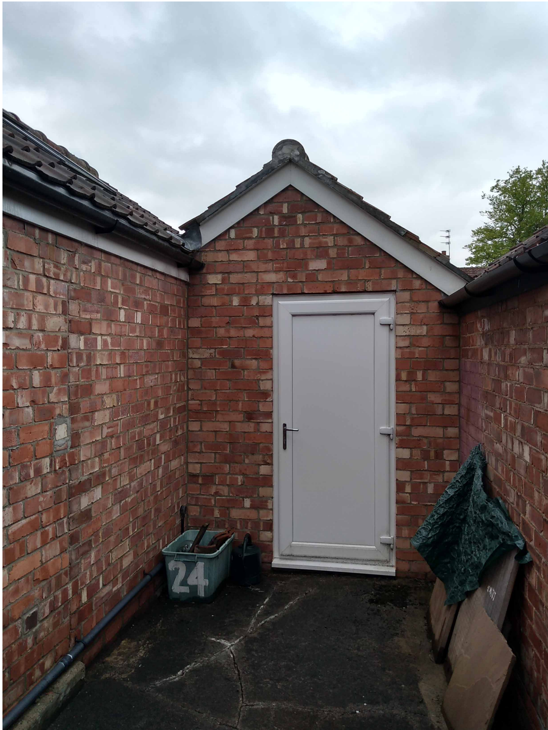
Photograph 5: Showing the front elevation of the garage and attached side elevation wall of existing extension. (Please see drawing number 6)
