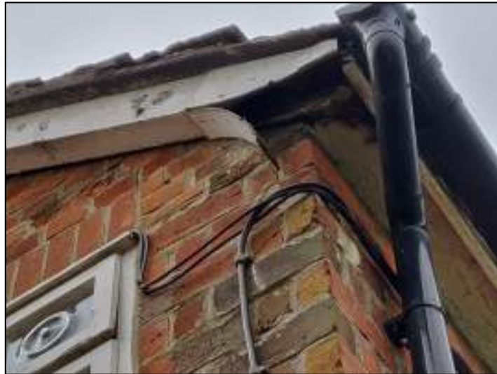
Photo 4.2: Building B1, rotten soffit on the northern corner of the building.
