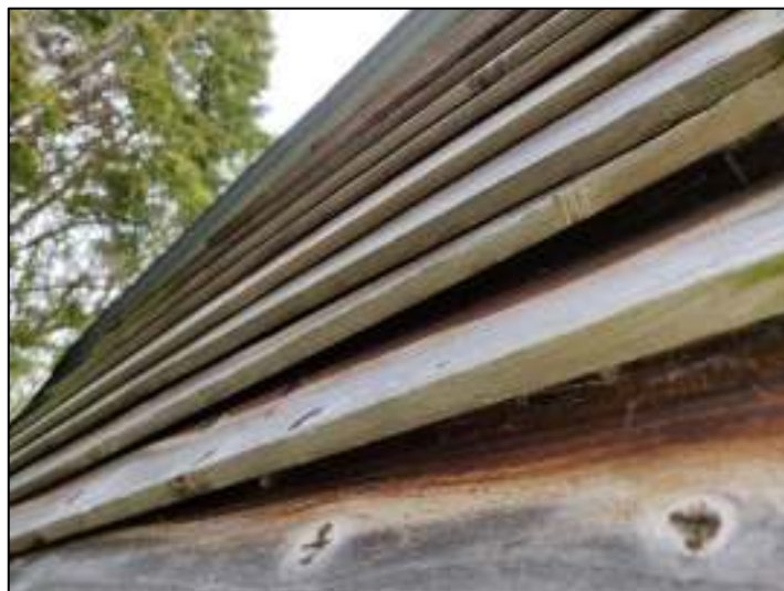
Photo 4.6: Building B2, gaps beneath the timber slats on the northern elevation.
