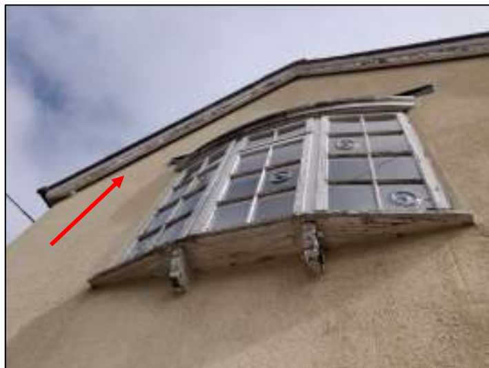
Photo 4.3: Building B1, gaps beneath the fascia on the south-western gable end (red arrow).
