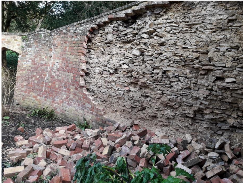
Photo 9: Summer House wall post 2021 collapse
