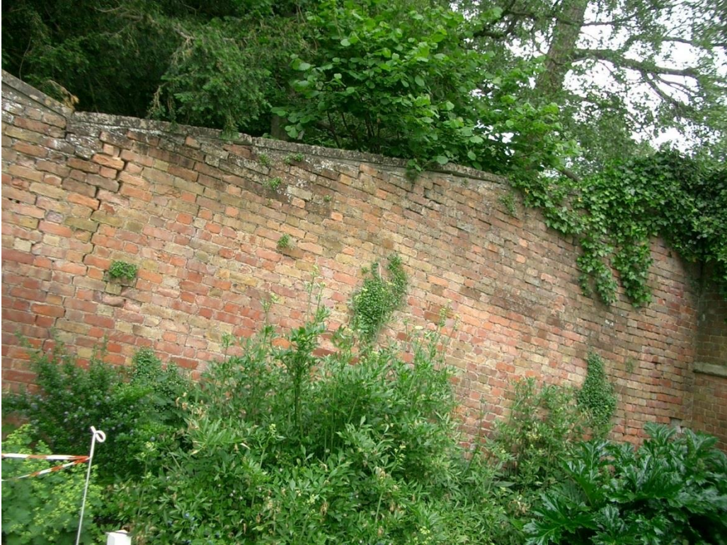
Photo 6: Summer House wall in early 2000s – cracking evident
