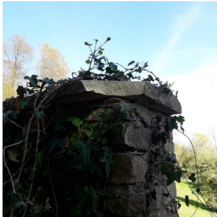
Broken Coping Section F (West end)
