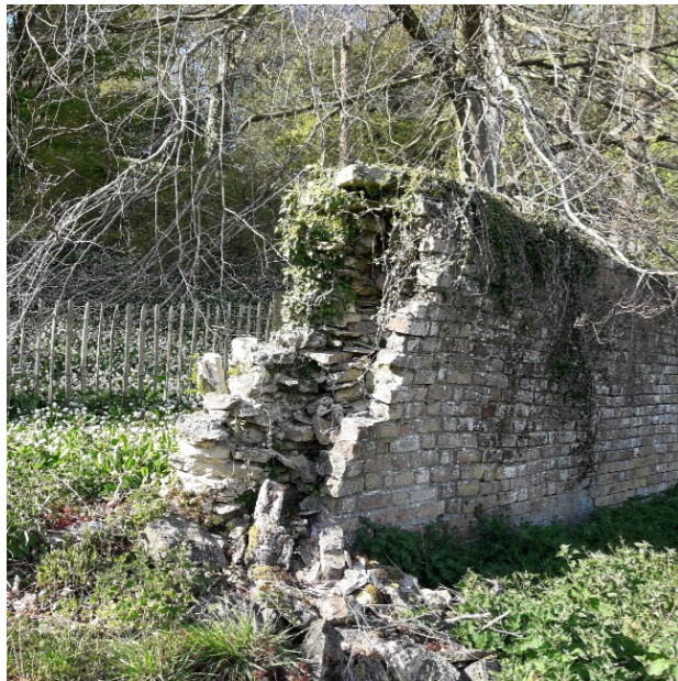
Collapsed wall at start of Section C
