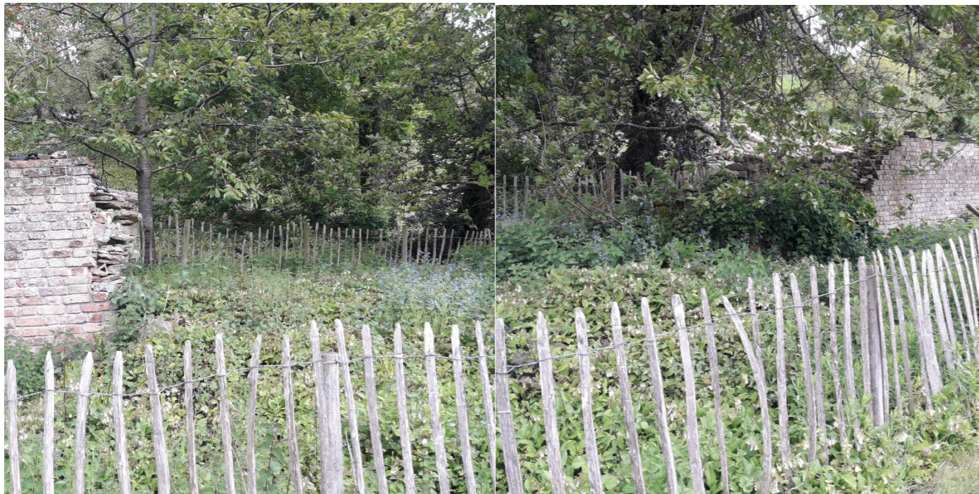
Section D – collapsed approx. 12.5m long
