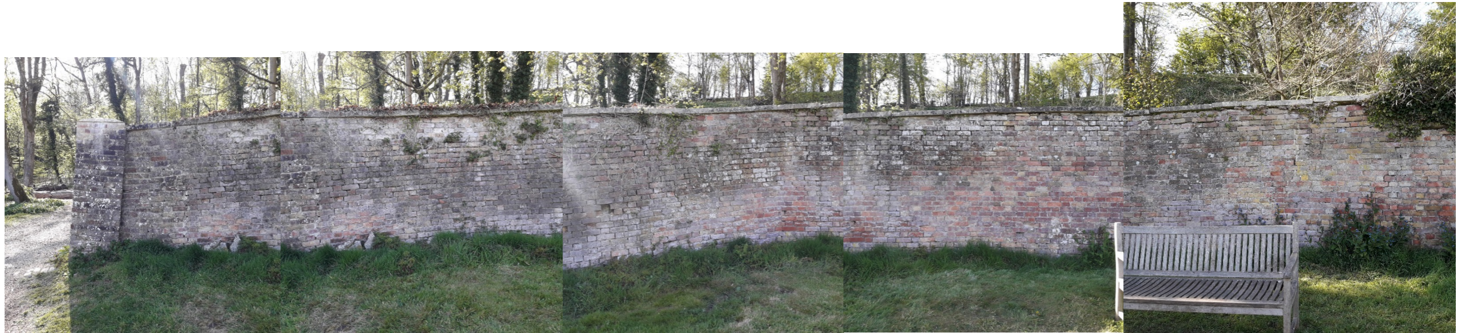
Section A (West to East): approx. 28m long and 2m to 2.5 high at front
