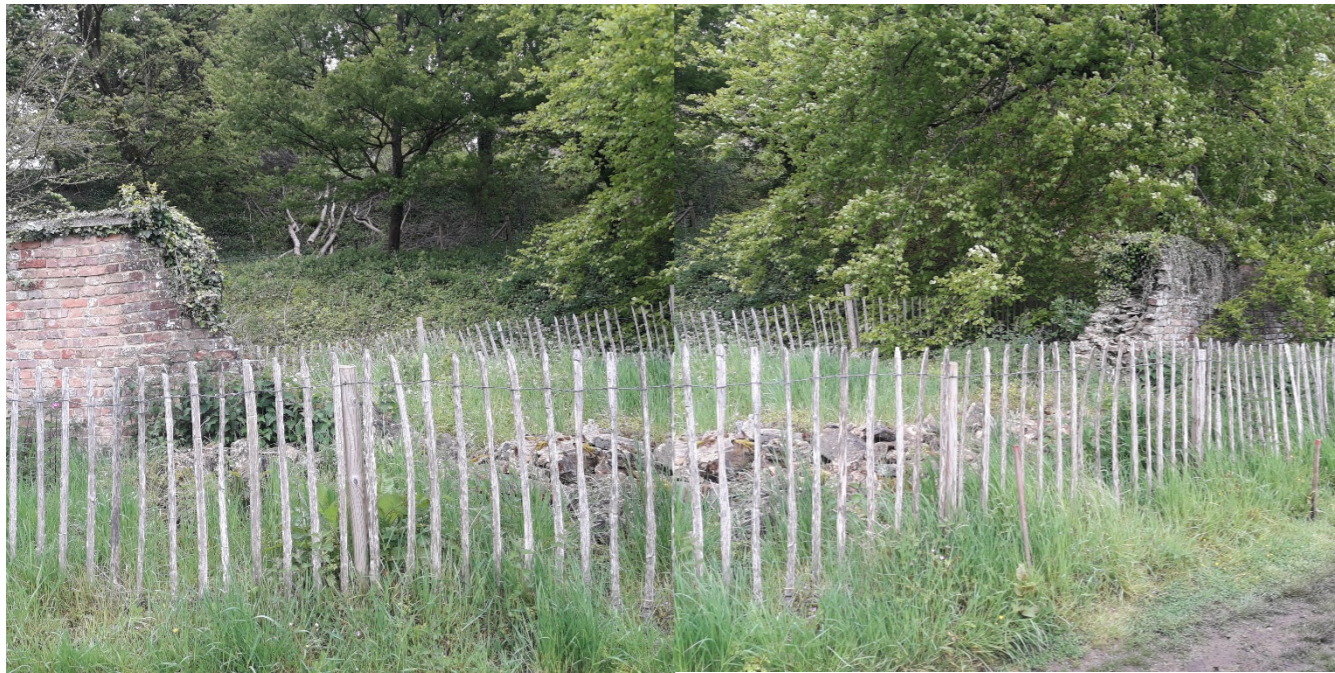
Section B – collapsed approx. 9.5m long
