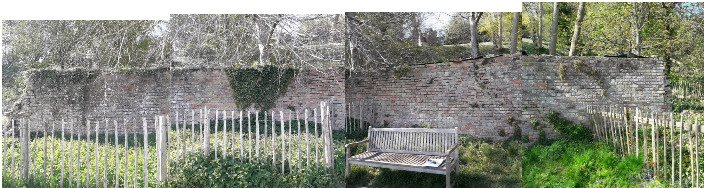
Section C (West to East): approx. 13.5m long and 2.25m high at front
