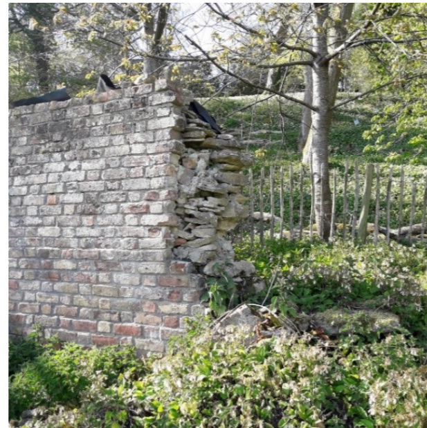
Collapsed wall at end of Section C
