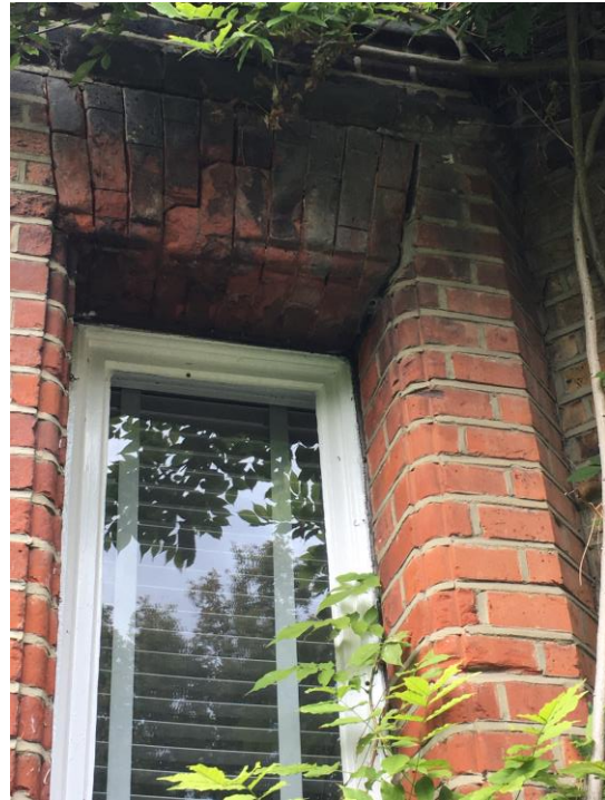
Missing mortar to brick arch
