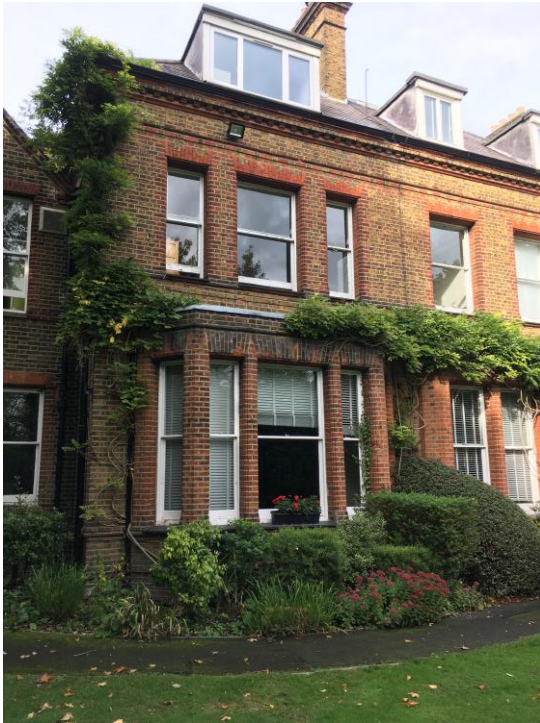
Affected front bay structure
