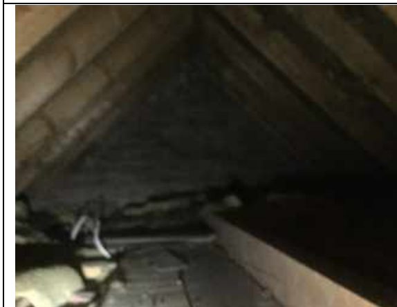
Photo 5 – Confined void above the extension on Wishanger Cottage.
