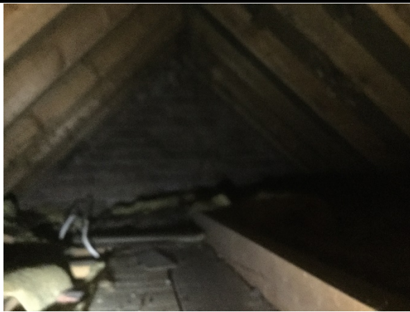
Photo 7 – Confined void above the extension on Wishanger Cottage.
