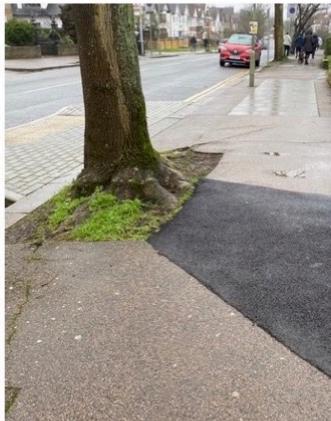
Tree T1, public highway tree as viewed in a southerly direction showing existing hard landscape updated to accommodate raised surfaces
