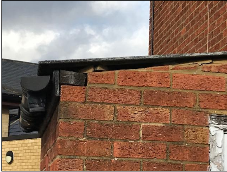
Photograph P Building B1 – Crevice under roof of small store structure at one end of the Presbytery
