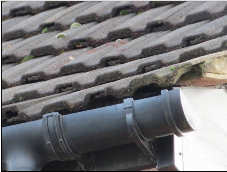
Photograph M Building B1 – Crevices present under roof tiles
