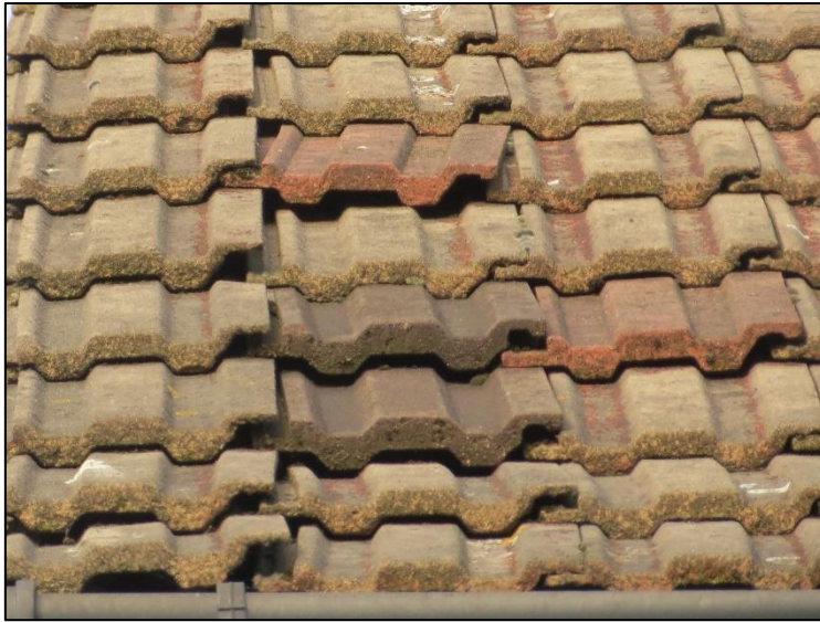
Photograph R Building B1 – Crevices noted under lifted and slipped roof tiles
