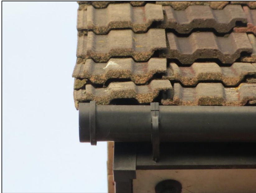
Photograph O Building B1 – Crevices present at corner of roof where there is a lifted roof tile
