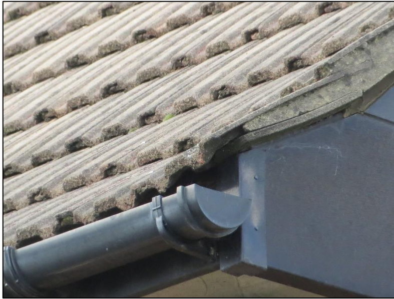
Photograph N Building B1 – Crevices present under further roof tiles
