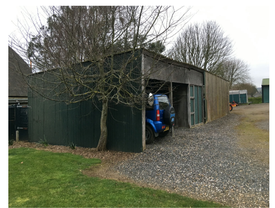
PHOTO SHOWING EXISTING STRUCTURE (In Poor Condition, & Unsuitable for Palletized Storage)
