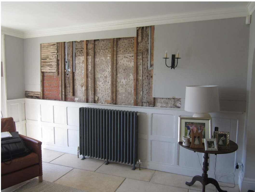
East face of wall between rooms G7 and G8, where it is proposed to make an opening.
