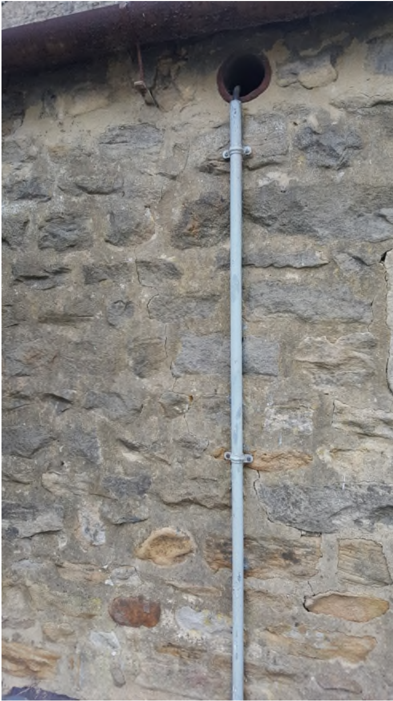
Minor cracking to right hand side – Wall 2
