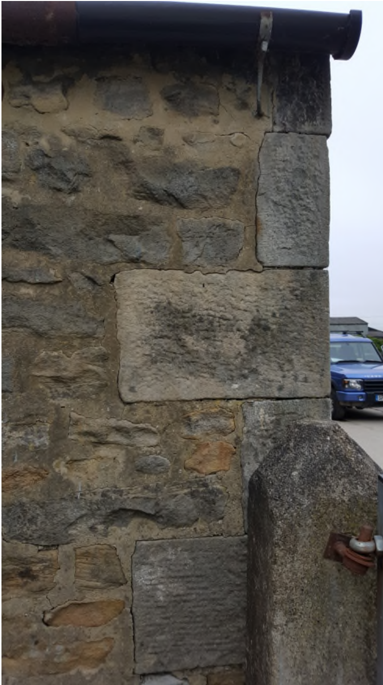
Minor cracking right hand side – Wall 2
