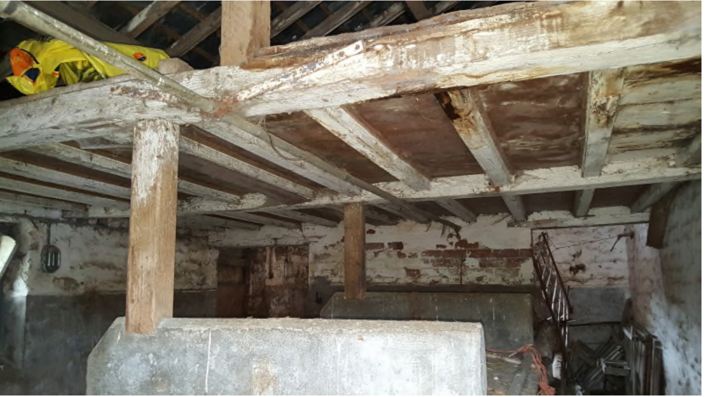
Internal – Single storey section – South elevation/Wall 2 Boarded area forming mezzanine type storage above
