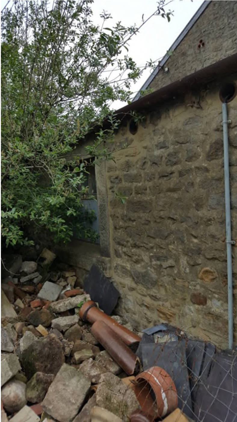
Outward movement to window and surrounding stone – Wall 2
