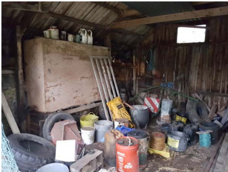
diesel tank in barn D, south of site
