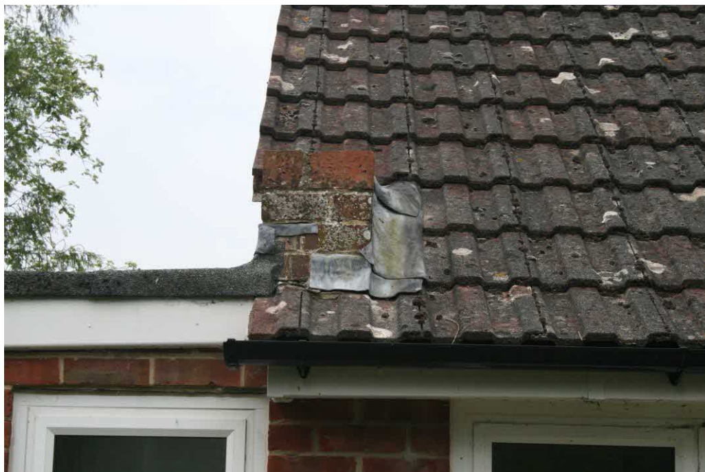
Figure 3: East elevation gaps in flashing
