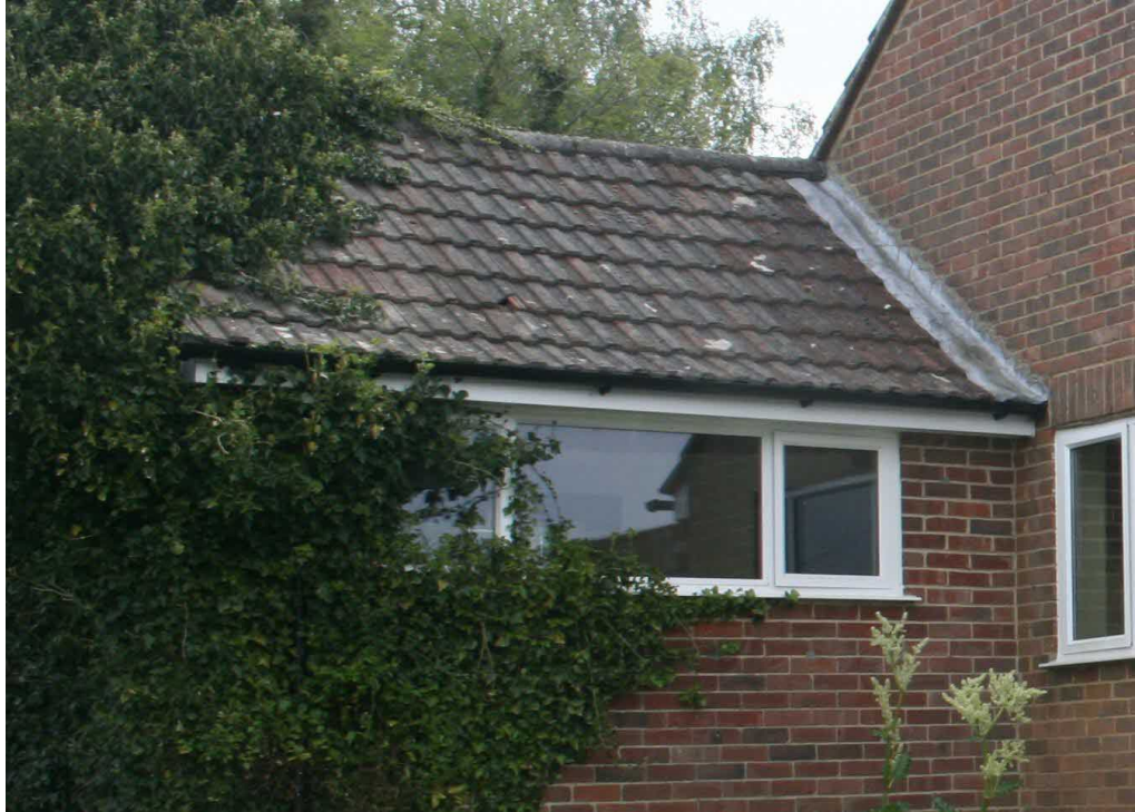
Figure 2: View of west elevation of bungalow, showing gap in tiles and partial ivy covering of roof on western roof pitch.
