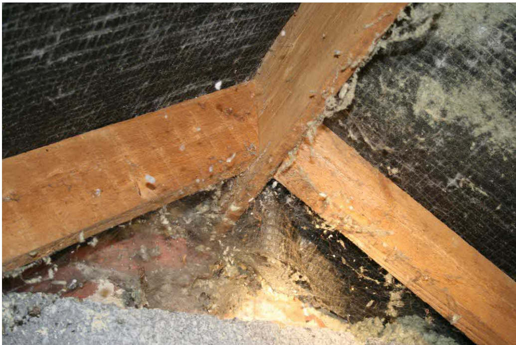
Figure 5: Gable End of roof space showing heavy cobwebbing
