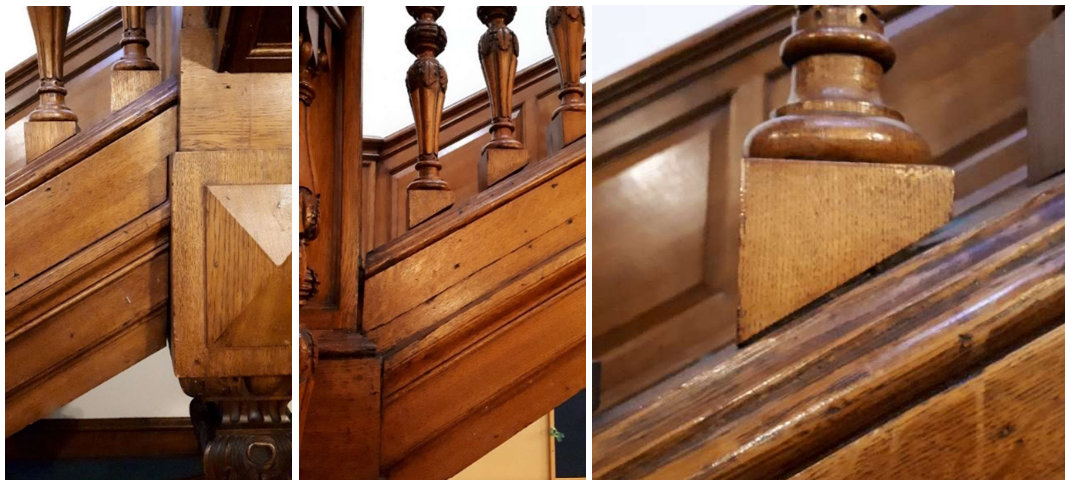
Figure 6: Evidence of movement in timber stringer and baluster connection. Note gaps at interface and at connection with post.
