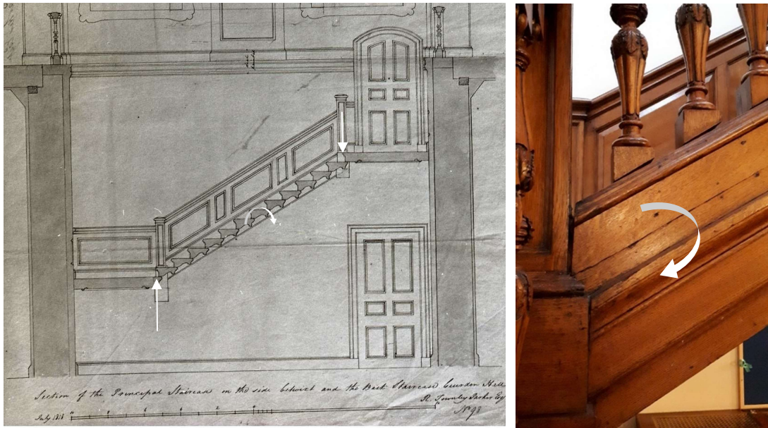
Figure 9: Evidence of movement with open joints between stringer and corner 'post'.
