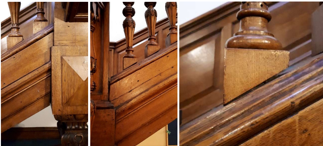
Figure 6: Evidence of movement in timber stringer and baluster connection. Note gaps at interface and at connection with post.
