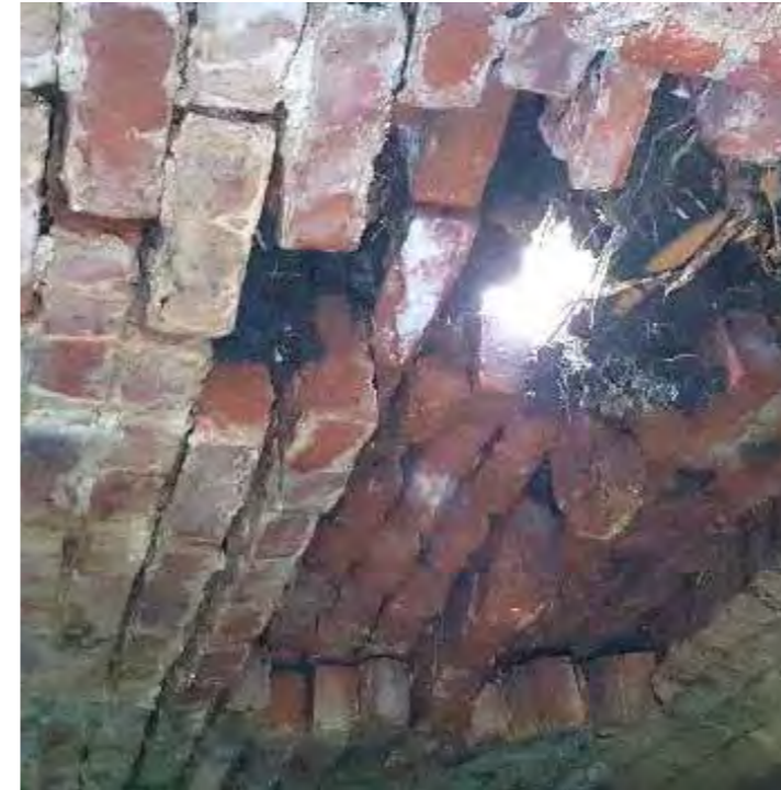
Above: Area of collapsed masonry units and hole through centre of the vault.
