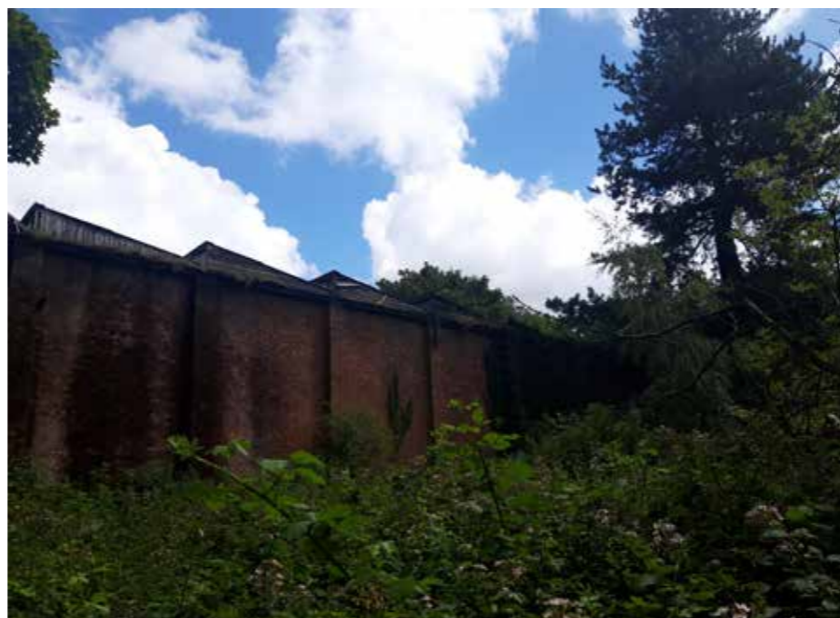
View of the unused and overgrown land between the west elevation of the stableyard and Cuerden Close.
