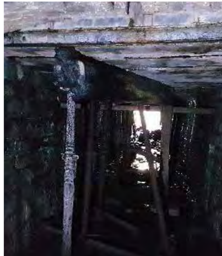
Above: Corroding acrow props installed below corroding steel and concrete filler joist deck below roadway.
