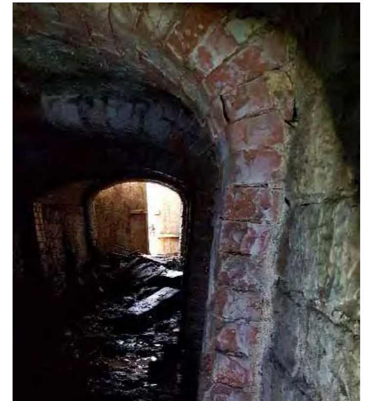
Above: Walls clearly spreading outwards, including relieving arches installed later and now also structurally compromised.
