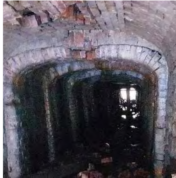
Above: Deformed masonry barrel vault with loose masonry units.
