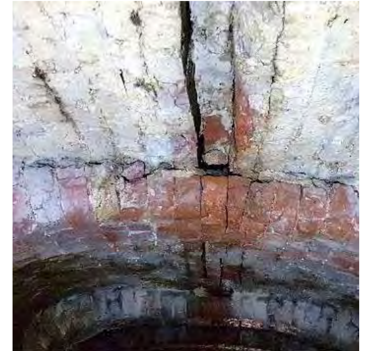
Above: Unbonded arches and thinner at crown indicates the relieving arches were installed later as an attempt to resolve the spreading and collapsing vault.
