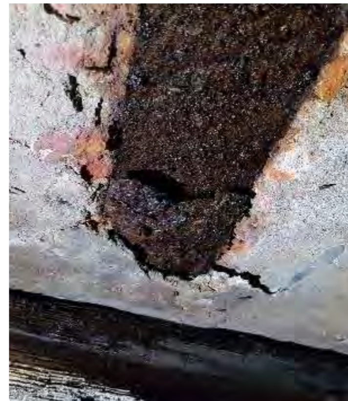
Above: Corroding filler joist beneath roadway.
