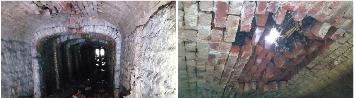
Figure 3: Deformed masonry barrel vault (left), and collapsed sections of vault with loose masonry units (right).
