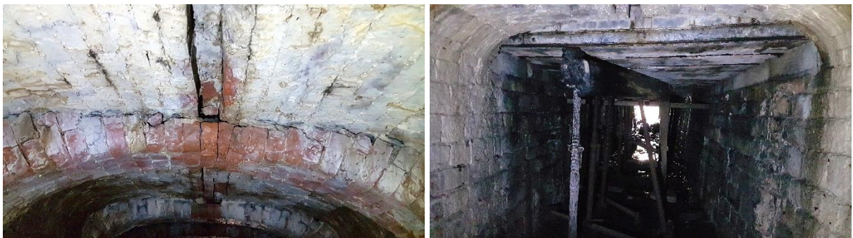
Figure 4: Arches unbonded and thinner at crown as if cut to fit deformed shape (left), and filler joist below road (right).
