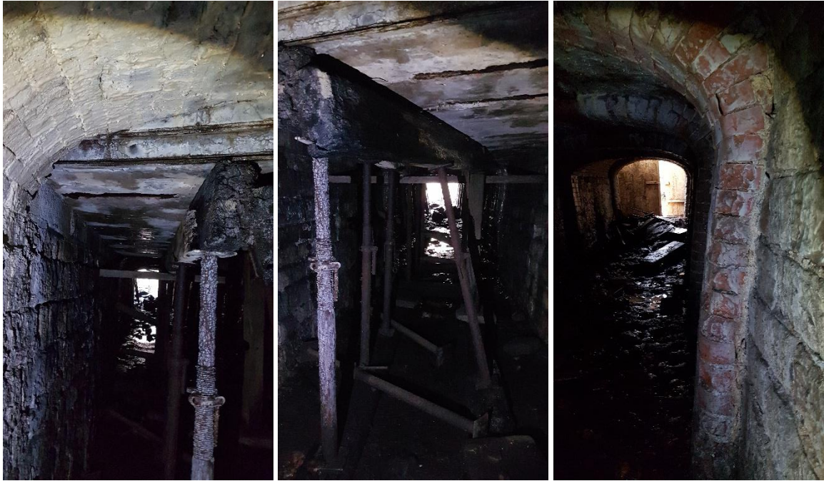
Figure 6: Filler joist section propped (left and centre), verticality of walls deformed (right).
