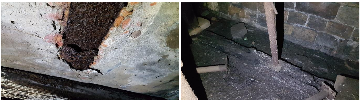
Figure 5: Concrete spalled and joists corroded (left), acrow props are corroding and the timber beams decayed (right).
