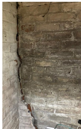
Brick built outbuilding in a state of disrepair and is to be demolished as part of the replacement studio proposals as permitted development
