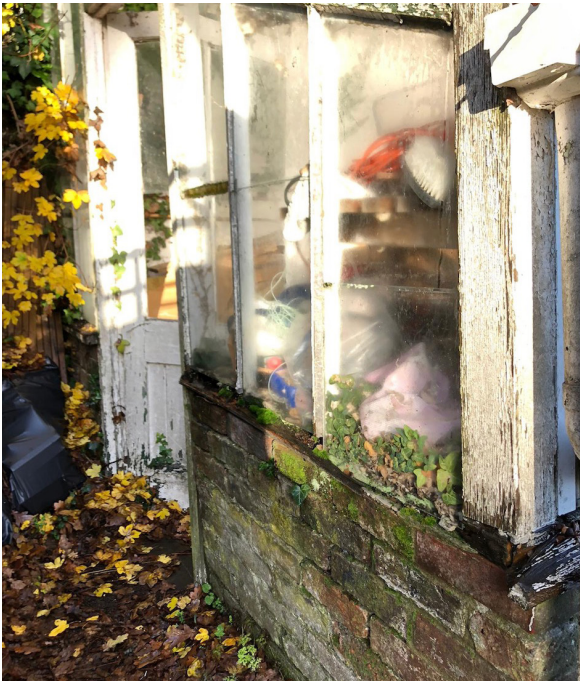
Existing timber and brick built glazed outhouse structure in a dilapidated state
