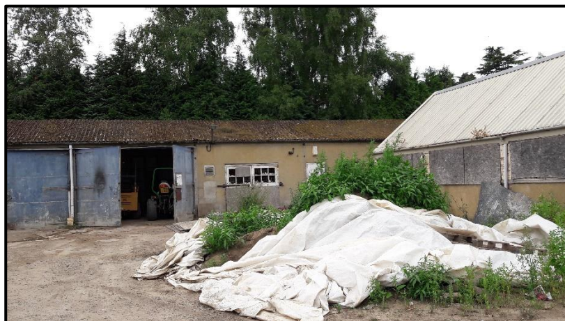
Photo 4.3: Building 2 – facing north-eastern and middle sections, with B3 to right of photo.
