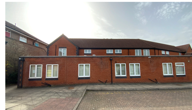
View over the existing rear flat-roof wing (foreground) and First floor administration accommodation (background).
