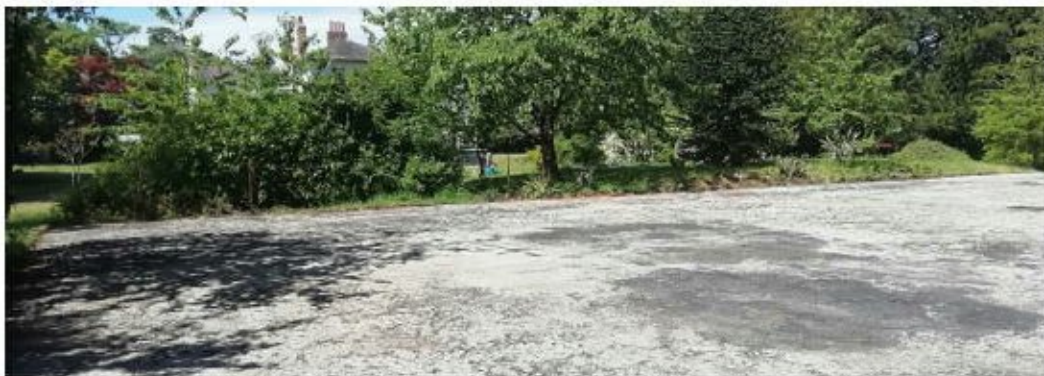
Fig 47 New, mesh fence to enclose derelict tennis court with new summer house to south
