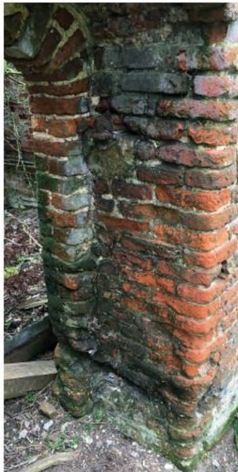
Figure 26: Existing jamb to be made good. New one to small gate to be similar
