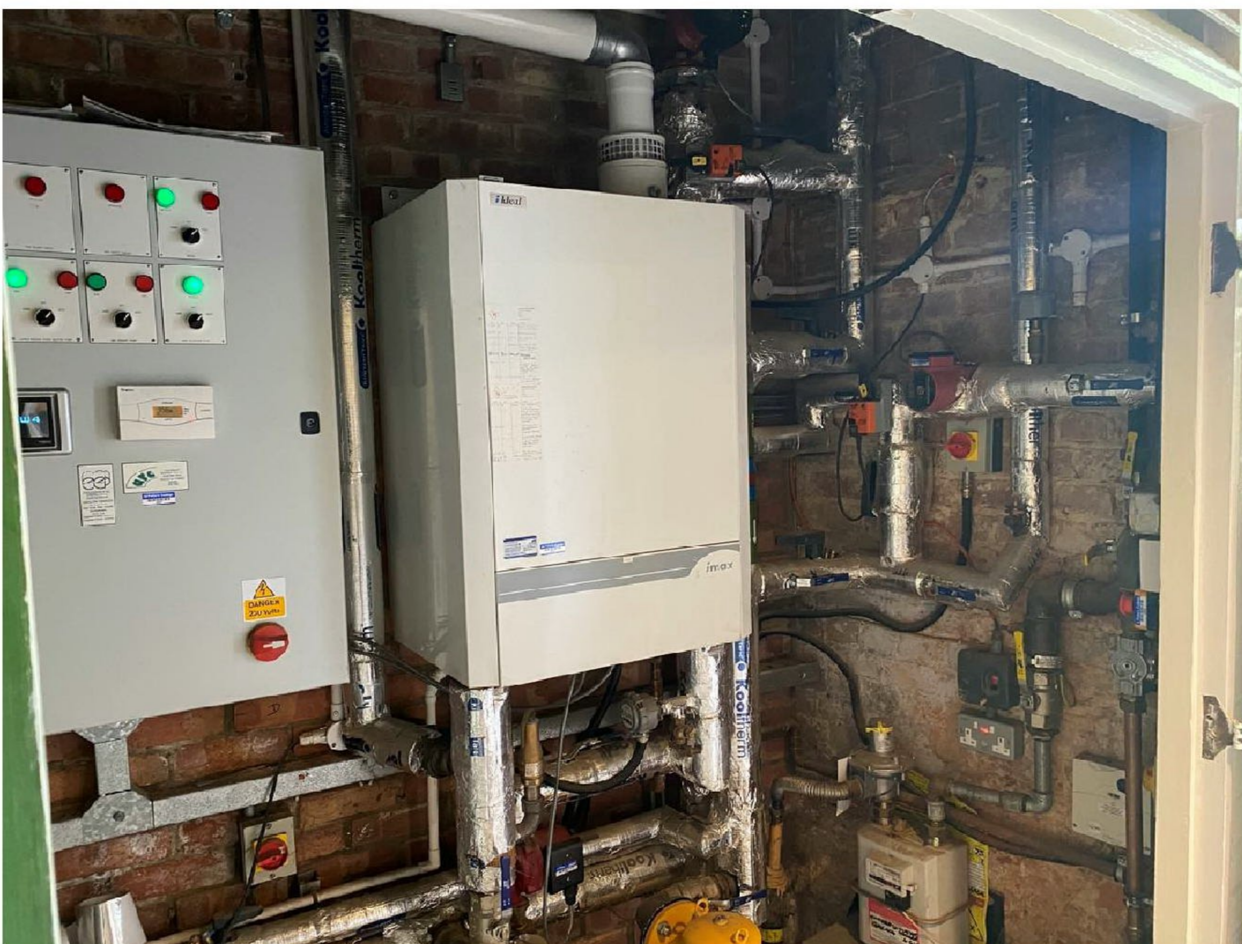
View of plant room showing existing boiler and connections at ground floor level.
