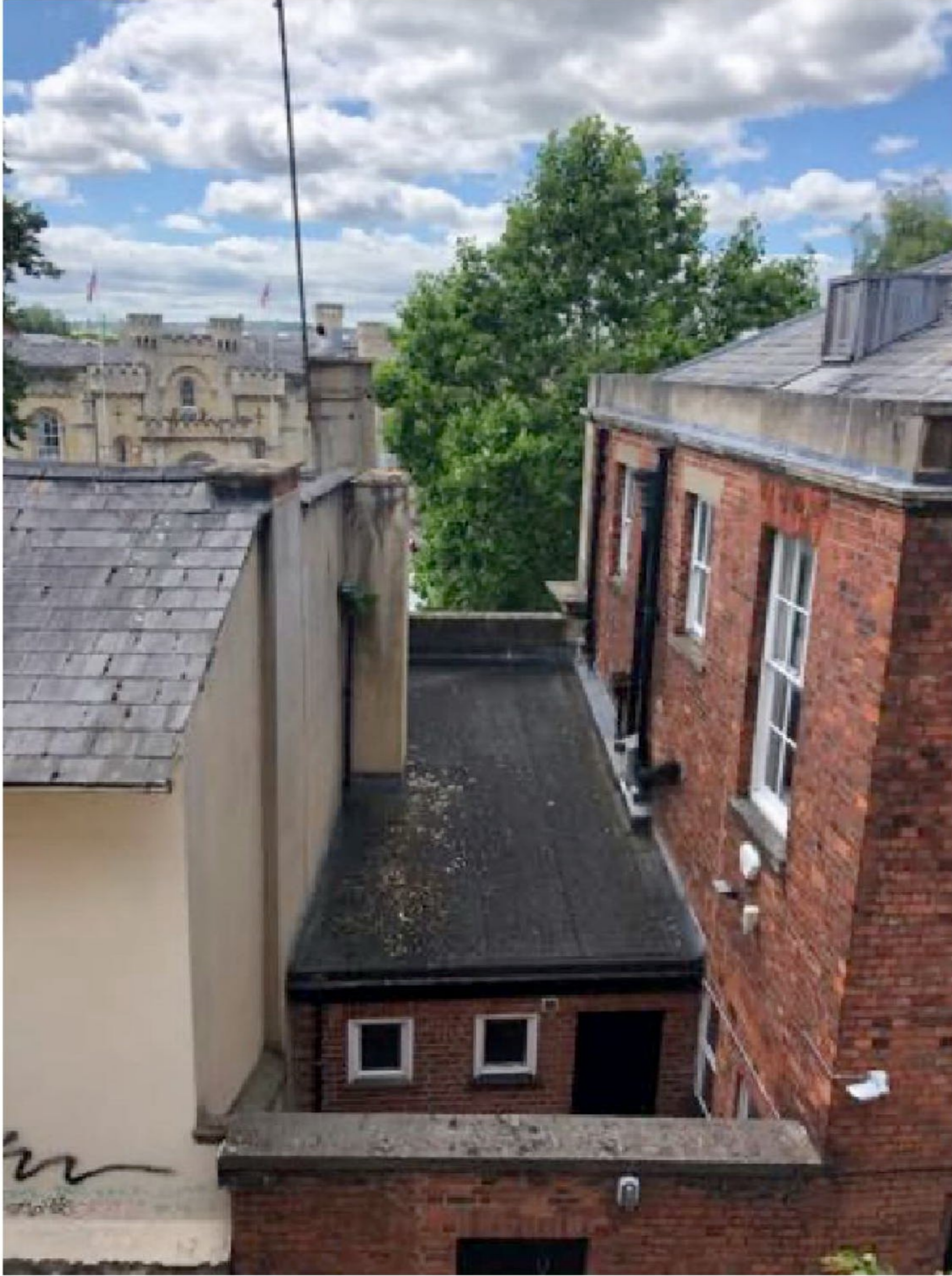
View of area of monopitch roof affected by the proposal, with Castle Hill House to the left and Canal House to the right.
