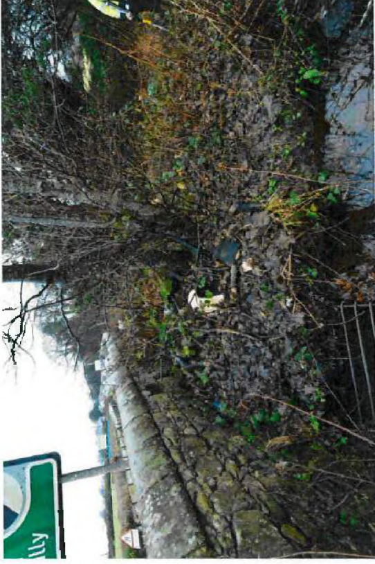
Plate 10: Watercourse at A78 culvert intake. Flow route during surcharge will be north into adjacent field (next plate). Photograph taken from NS 21040 96283.
