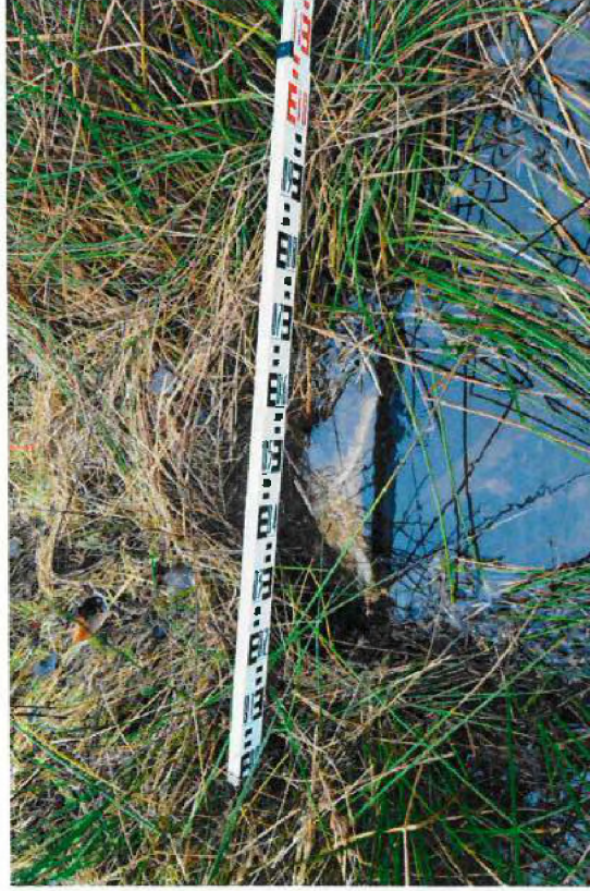
Plate 12: Culvert outfall (ID: 0.55 m H x 0.7 m W elliptical VCP pipe). Photograph taken from NS 21022 56294.
