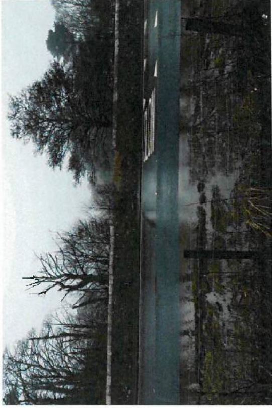
Plate 6: Looking east towards the source of the water pooling on the A78. The break in the wall was caused by a car crash. The field behind the wall is poorly drained and run-off flows onto the road. Photograph taken from NS 21035 56338.
