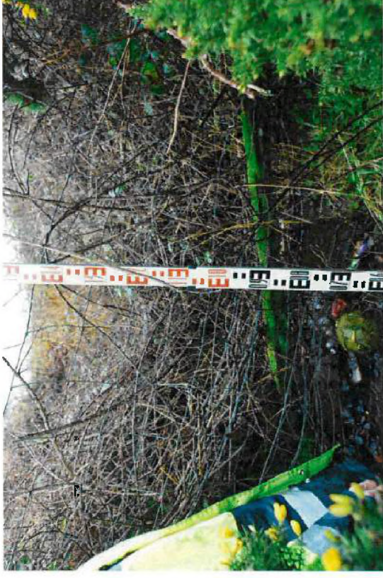
Plate 17: Channel of subject watercourse in front of railway line culvert. Photograph taken from NS 20985 56296 looking downstream.
