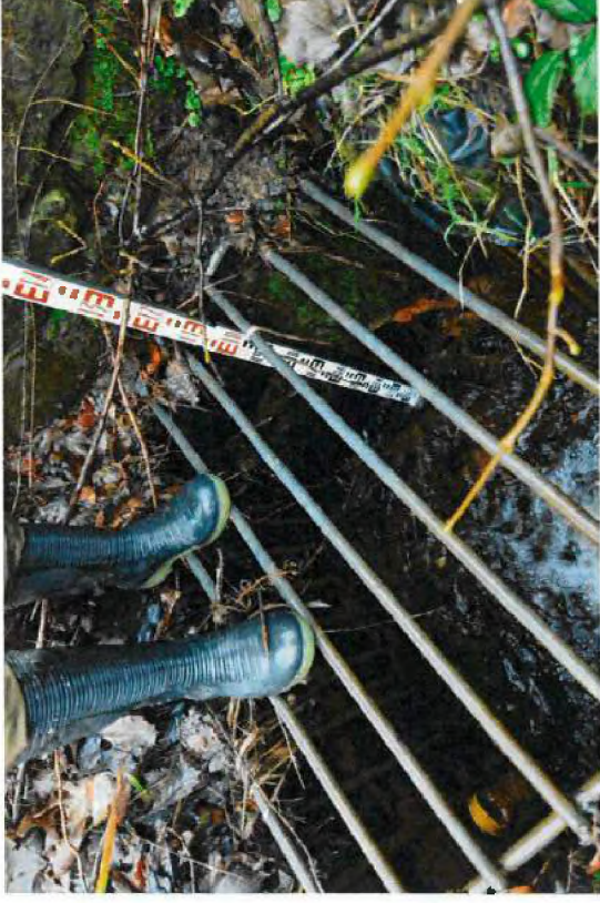
Plate 9: A78 culvert intake (0.55 m ID pipe with corrugated inner walls and wash screen with circa 100 mm spaced bars). Top of wall is c. 2.2 m above screen. Photograph taken from NS 21040 56284.
