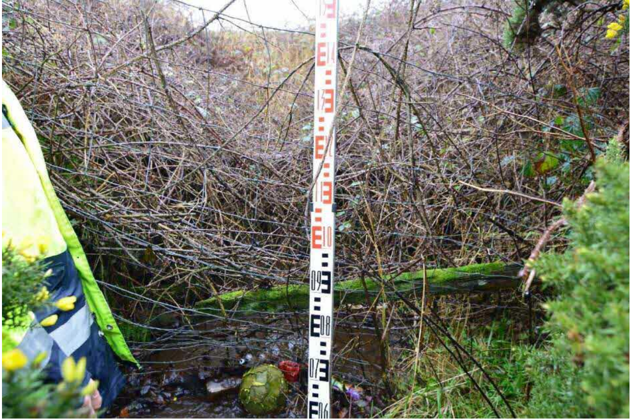
Plate 17: Channel of subject watercourse in front of railway line culvert. Photograph taken from NS 20965 56296 looking downstream.
