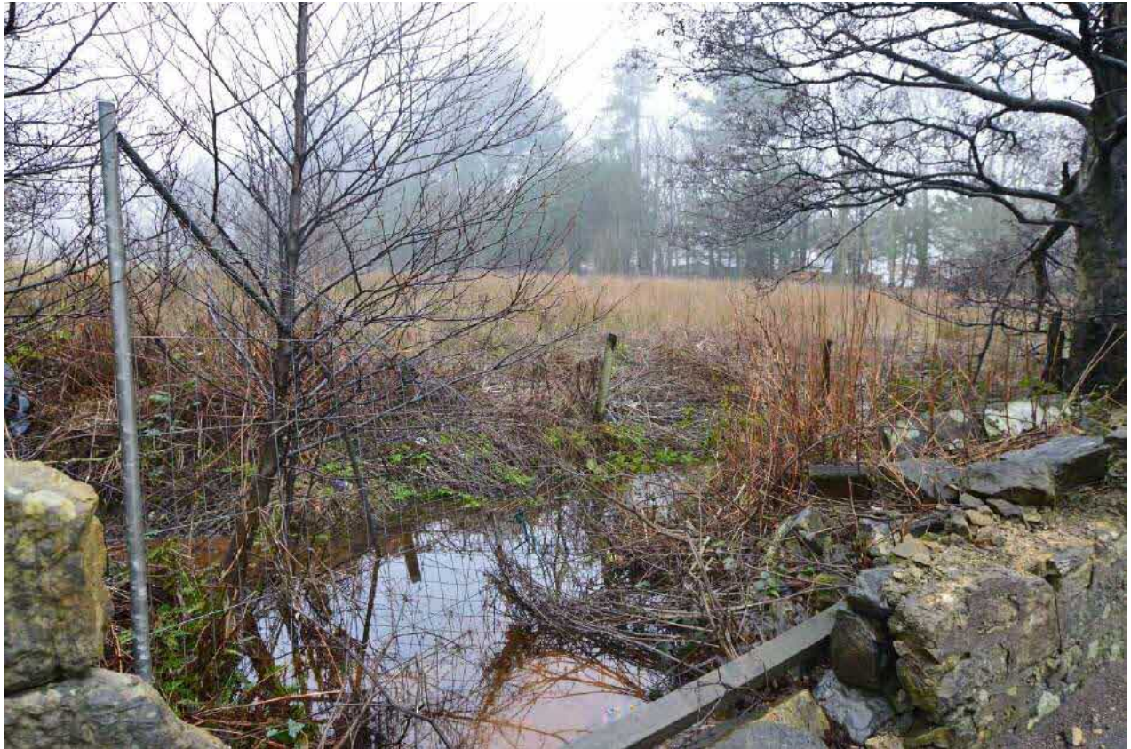
Plate 7: Source of A78 flooding. Photograph taken from NS 21050 56336.
