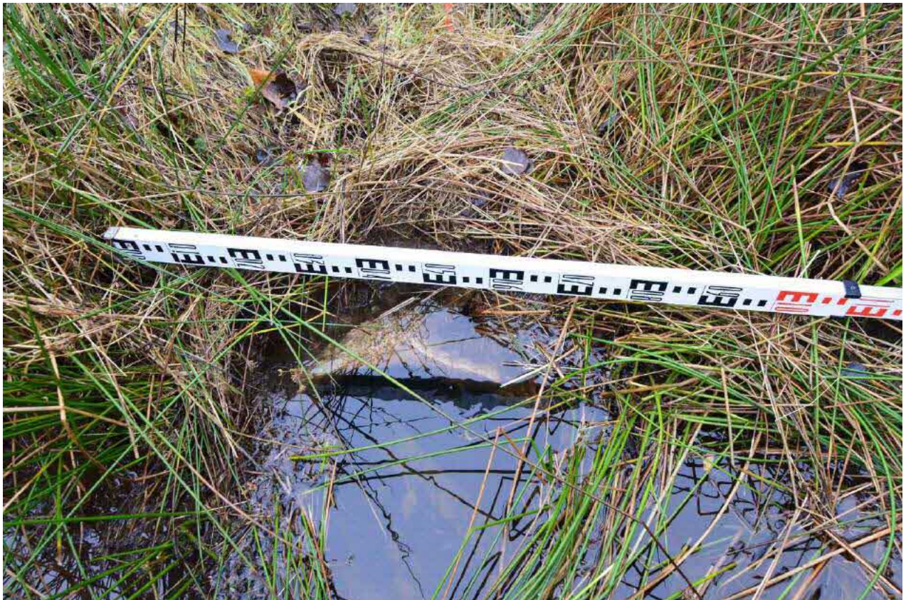
Plate 12: Culvert outfall (ID: 0.55 m H x 0.7 m W elliptical VCP pipe). Photograph taken from NS 21022 56291.
