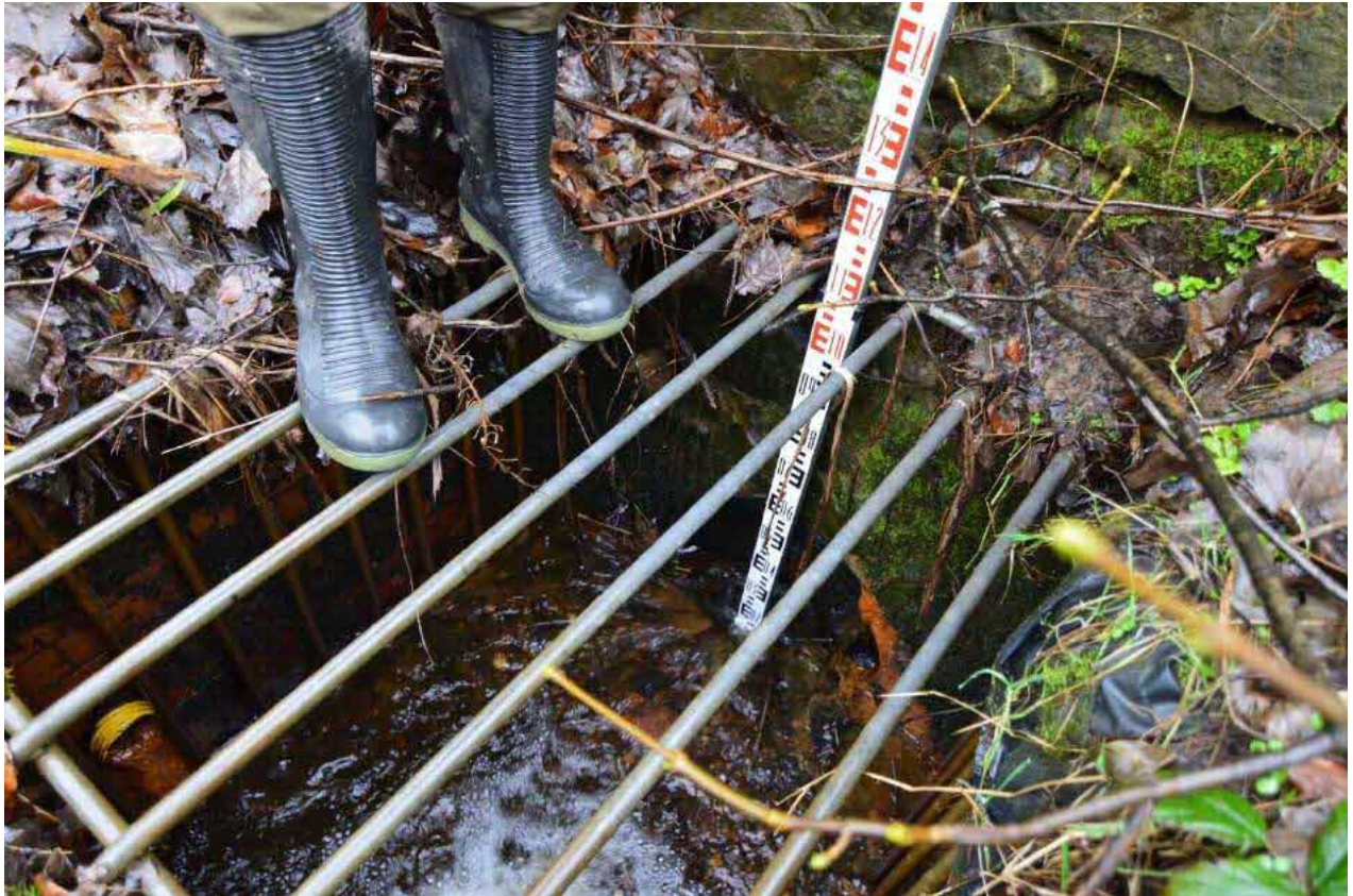
Plate 9: A78 culvert intake (0.55 m ID pipe with corrugated inner walls and trash screen with circa 100 mm spaced bars). Top of wall is c. 2.2 m above screen. Photograph taken from NS 21040 56284.
