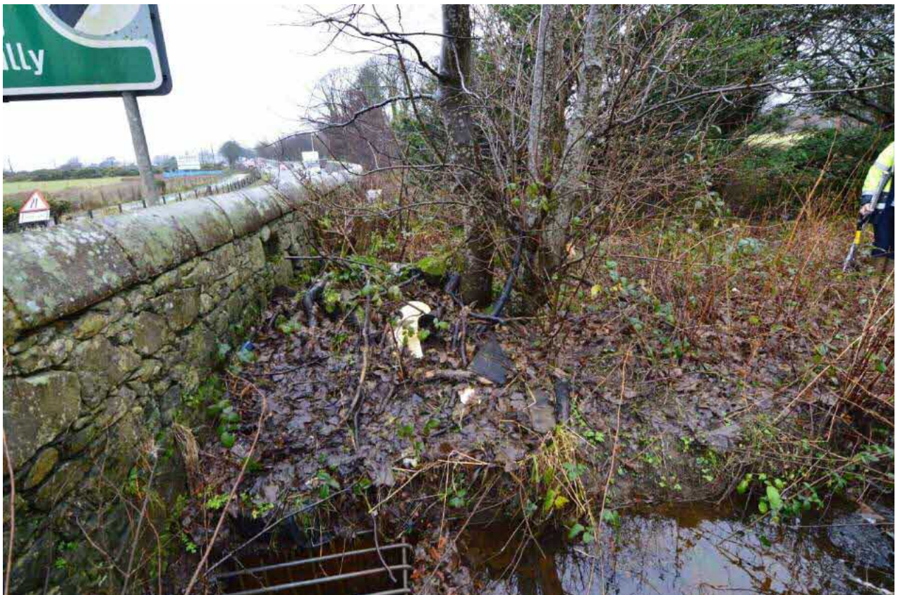
Plate 10: Watercourse at A78 culvert intake. Flow route during surcharge will be north into adjacent field (next plate). Photograph taken from NS 21040 56283.
