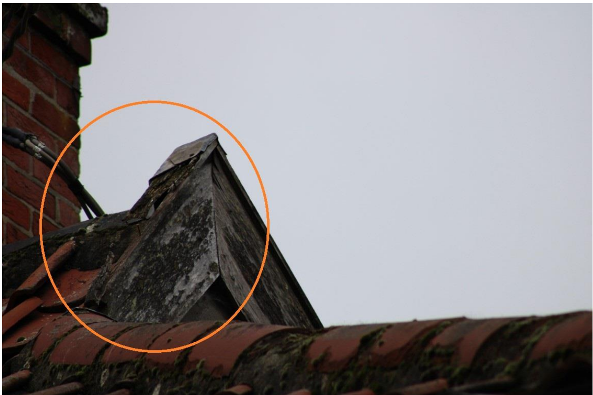
The front roof, rotted timber trim.
