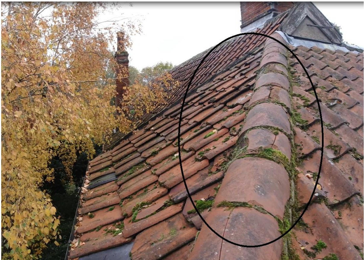
Damaged hip tiles to the front roof.
