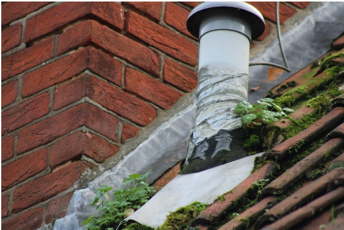
The taped up damaged soil vent pipe, and debris.
