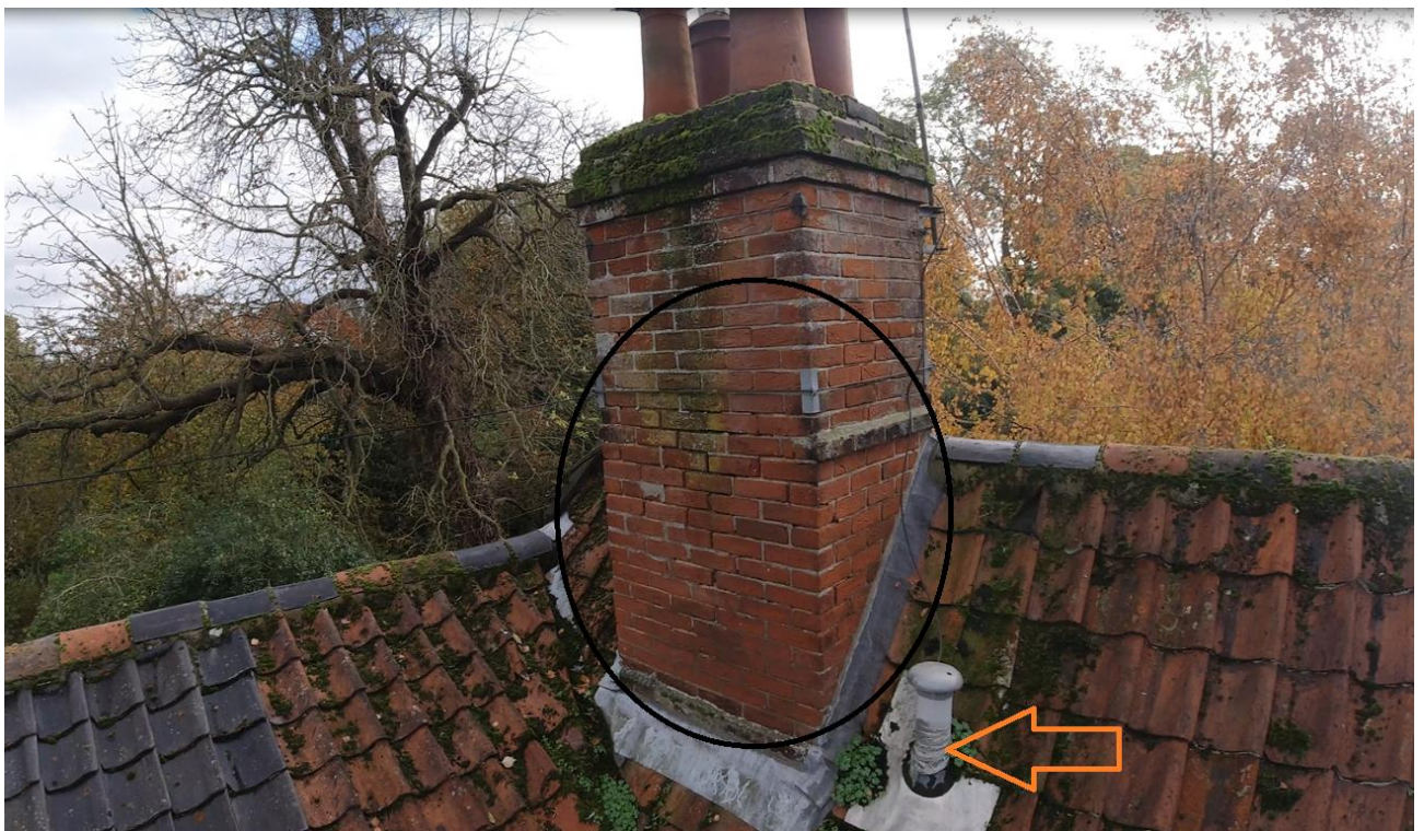
The chimney stack from the rear, and the damaged soil vent pipe.
