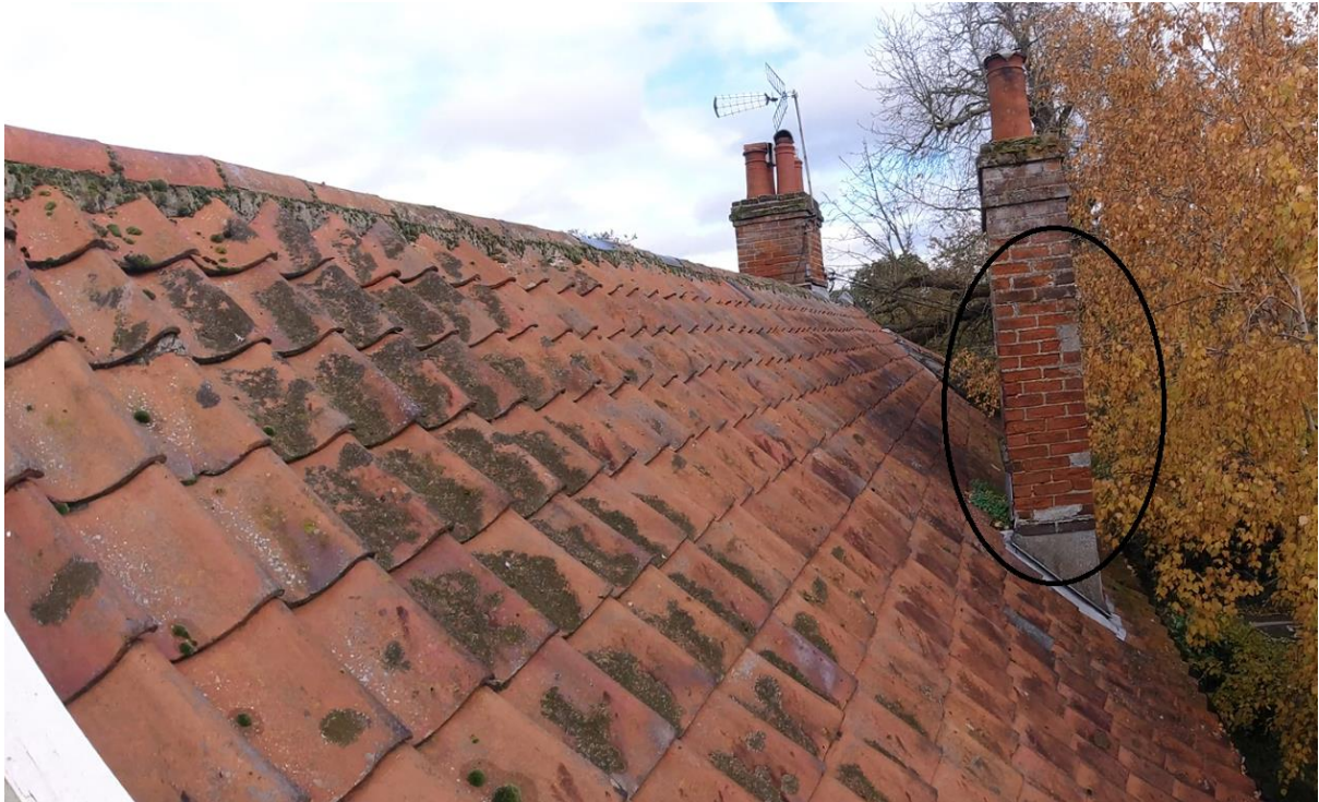
Concrete infill to the rear chimney stack, due to weathered faces to the bricks.
