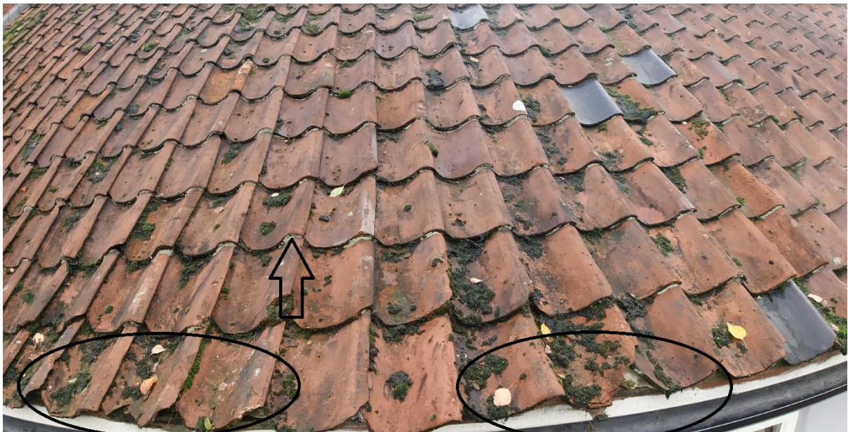
Damaged tiles to the rear roof. The arrow indicate the remains of mortar applied to the lower edges of the tiles as an attempt to reduce draughts under the tiles.
