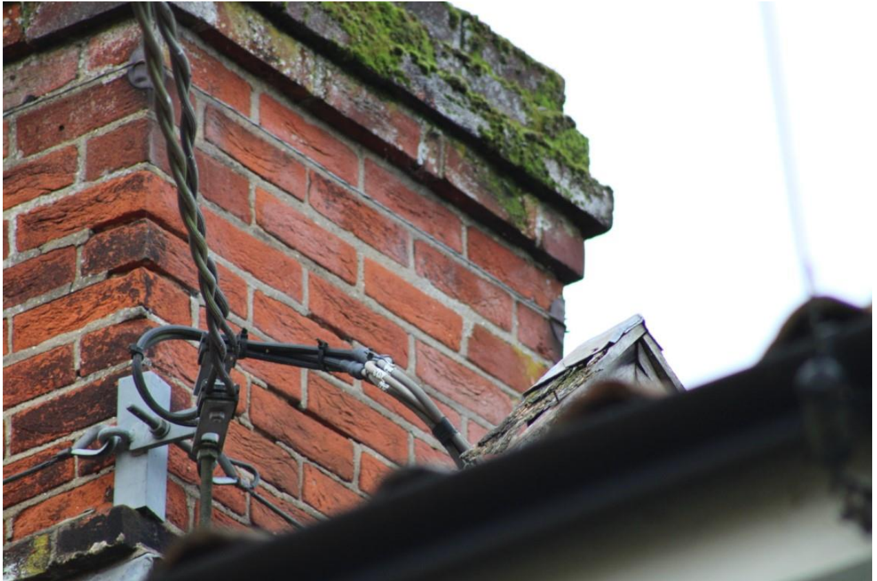
The front chimney stack viewed from the front, cement pointing between the bricks.
