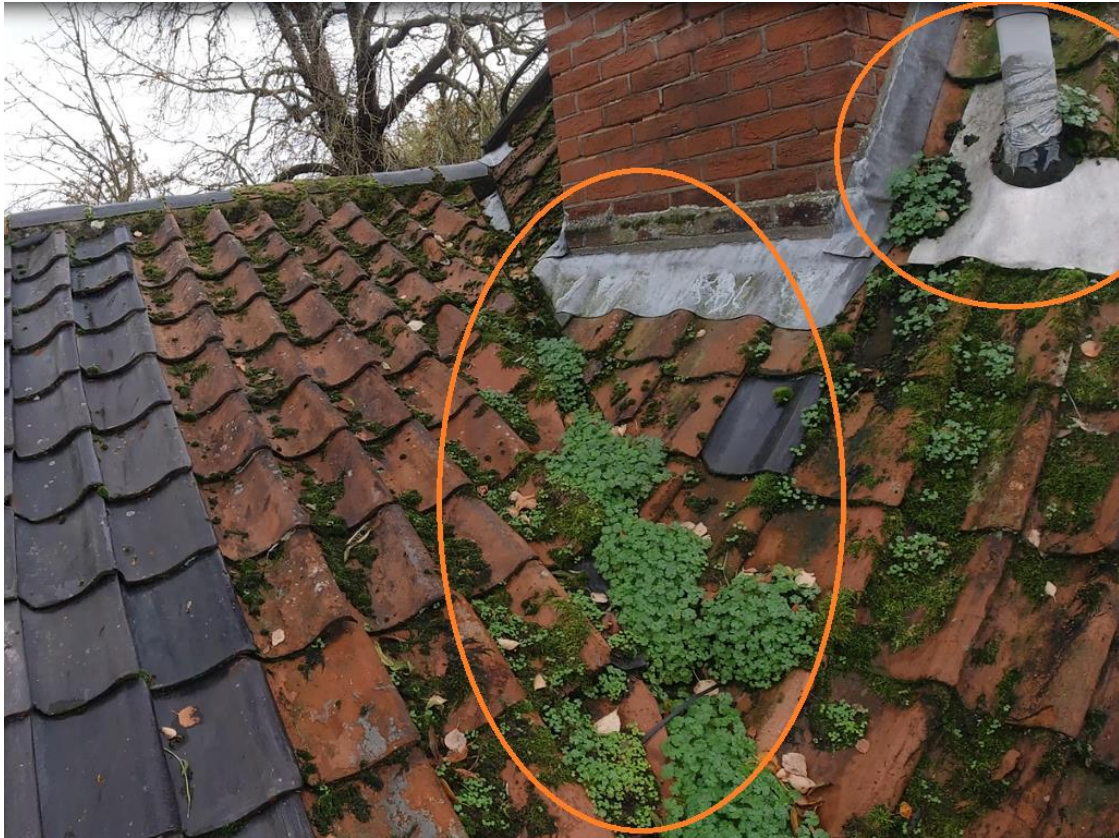
Debris to the roof valley.
