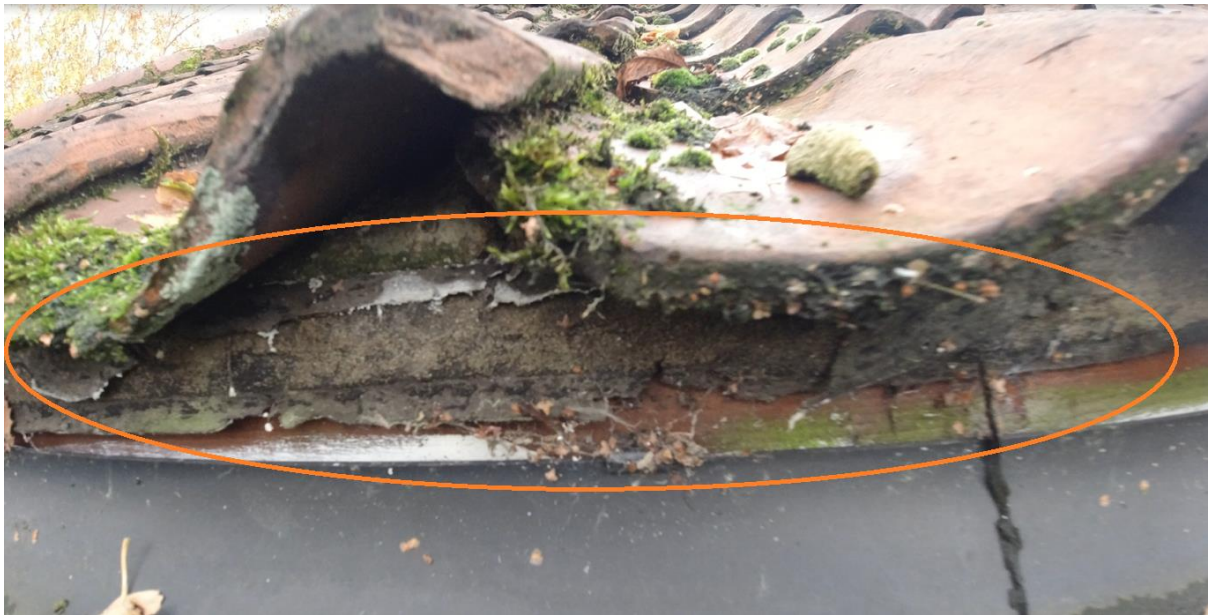
Damaged tile and rotted underlay to the front roof.
