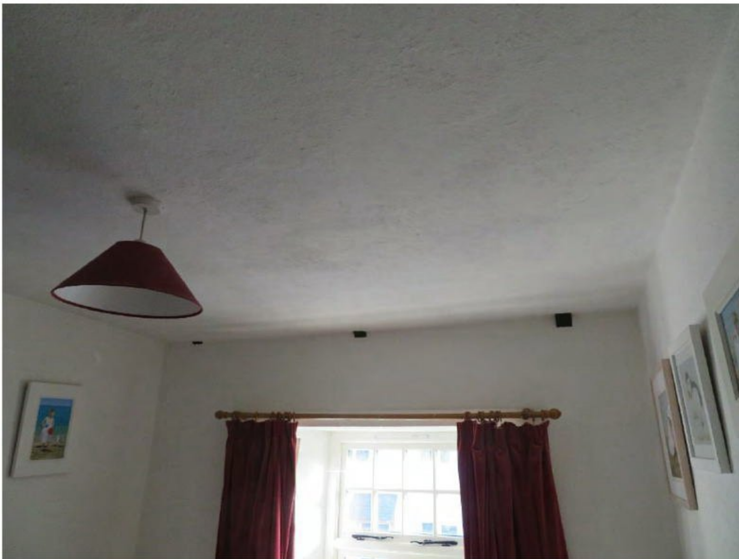
Photo 8 Internal view of northern section of east wall, note three roof trusses
