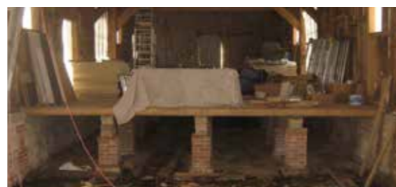
Photo taken recently on site showing the brick piers supporting the raised floor of the Granary (bays 4+5)
