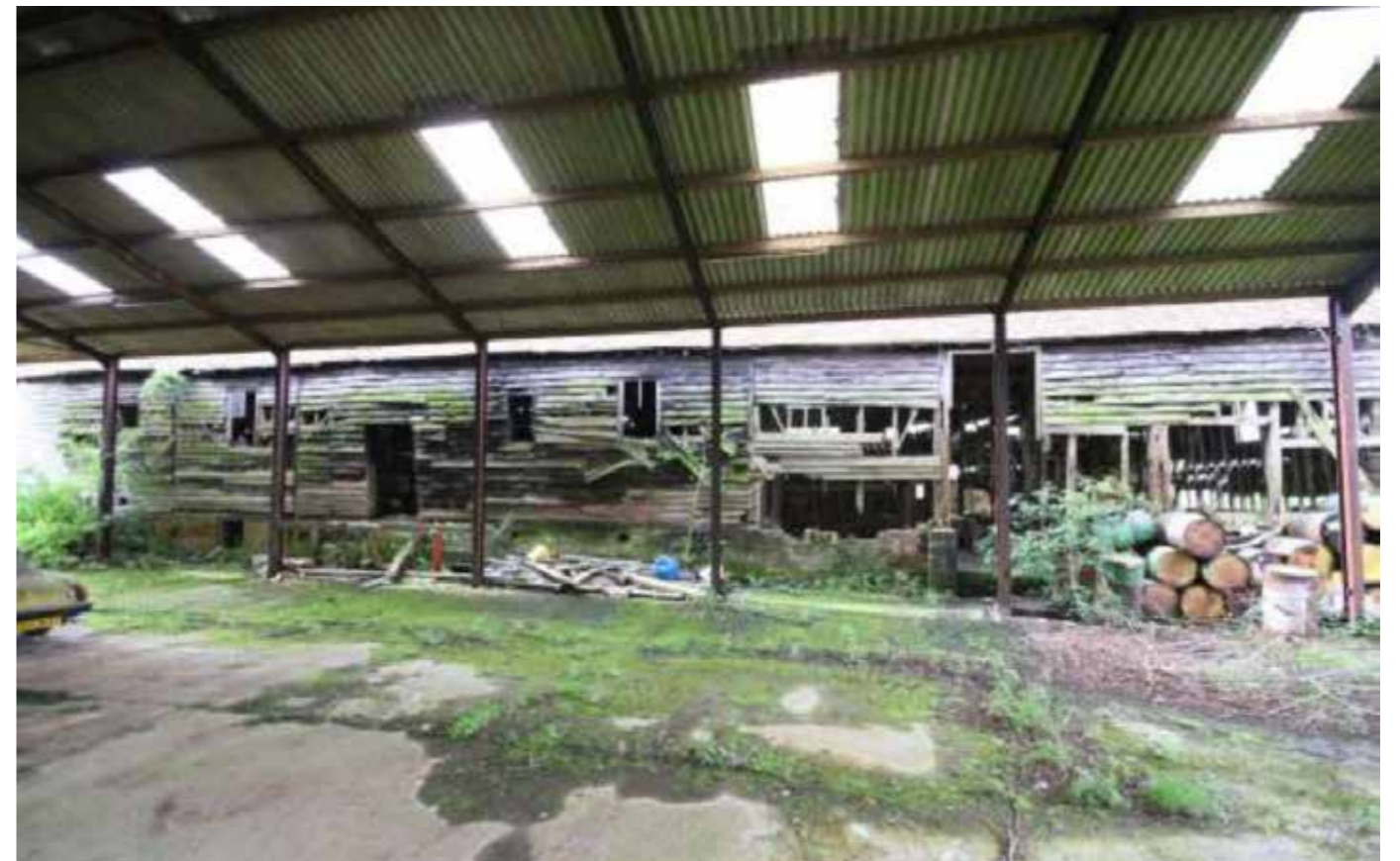
Photo taken from the approved scheme heritage report showing the poor condition of the Granary Building from within the atcost barn
