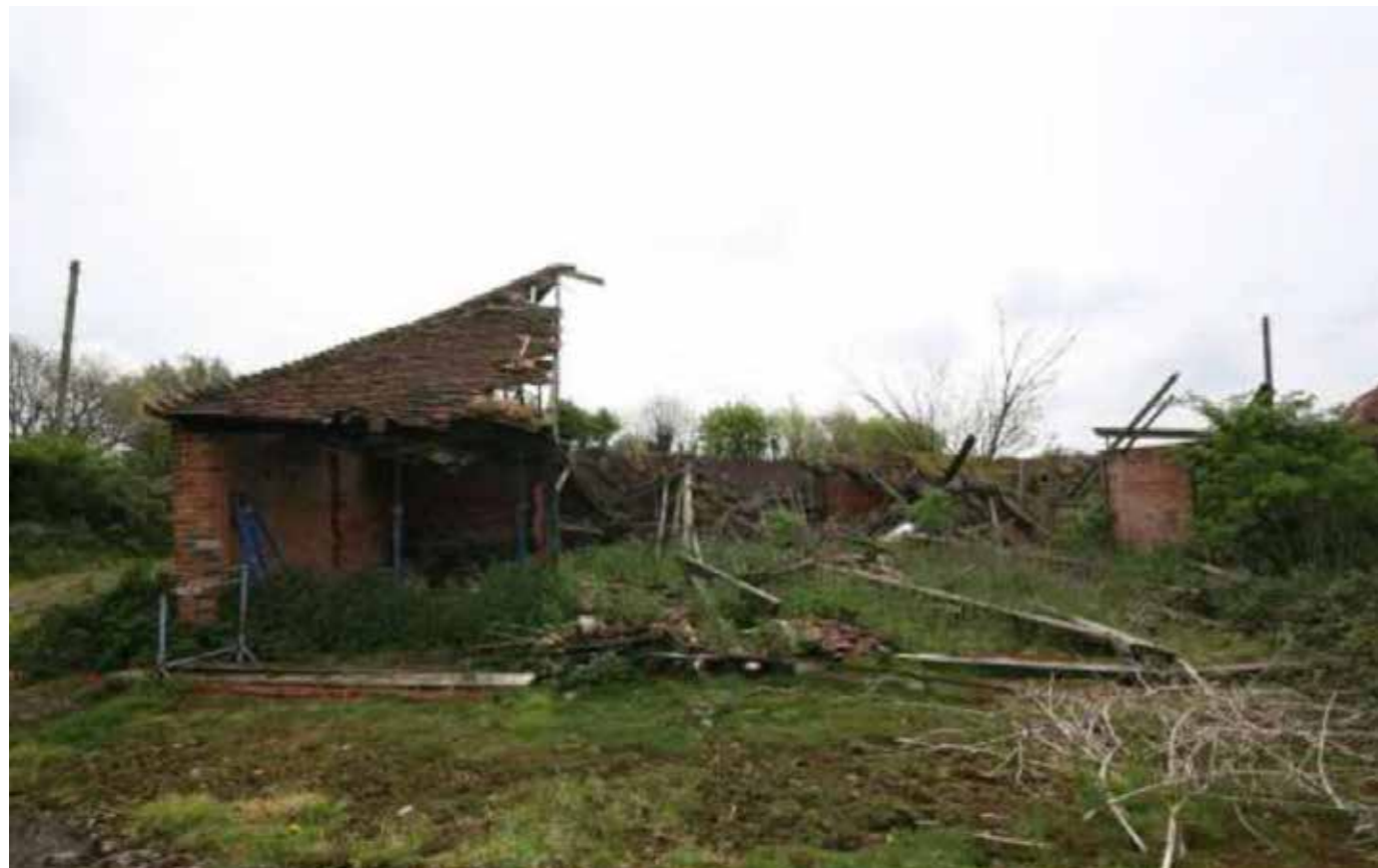
Photo taken from the approved scheme heritage report showing the poor condition of the Machine Shed
