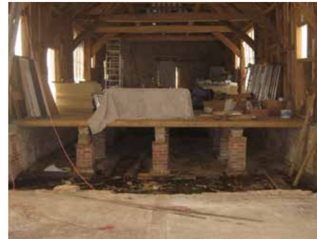
Brick Piers holding up the later added floor in bays 4 + 5. The proposal removes the central aisle of piers and the flooring, and would retain the left and right aisles of piers to be accommodated within the proposed scheme.
