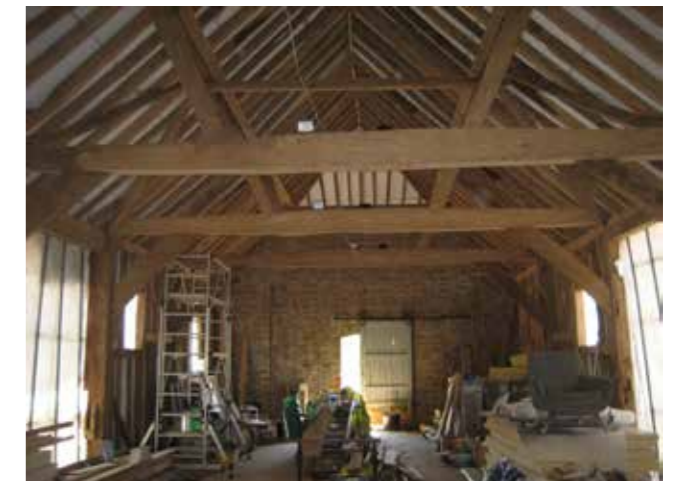
Additionally with this arrangement the south internal elevation unique brickwork would be revealed full height
