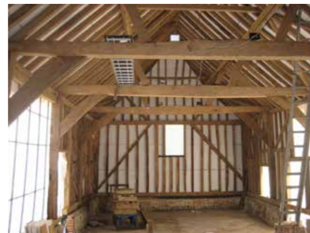
With this arrangement the north internal elevation timberwork would be revealed full height
