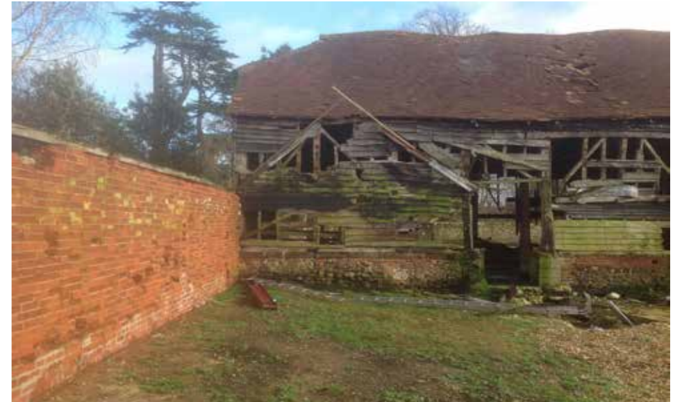
Photo capturing the zinc flashings still evident where the Link Building touched the Granary building
