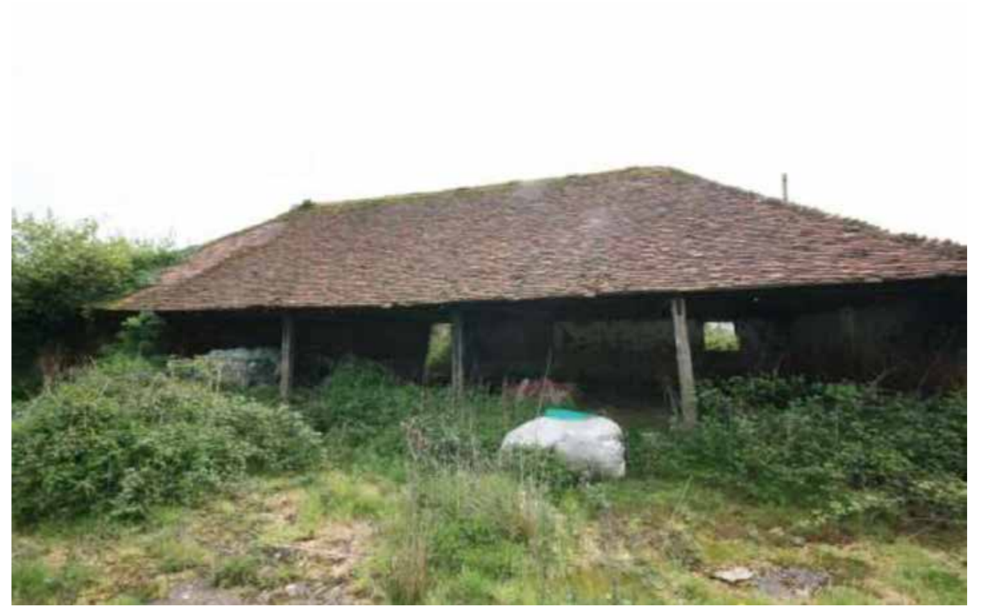
Photo taken from the approved scheme heritage report showing the poor condition of the Cart Shed
