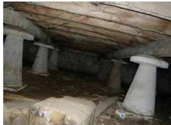
Photo taken from the approved scheme heritage report showing the concrete staddle stones (bays 1+3)
