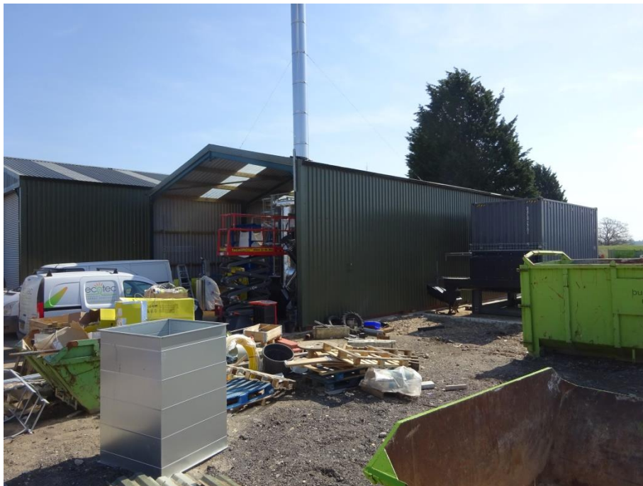
Non-Enclosed Boiler House
