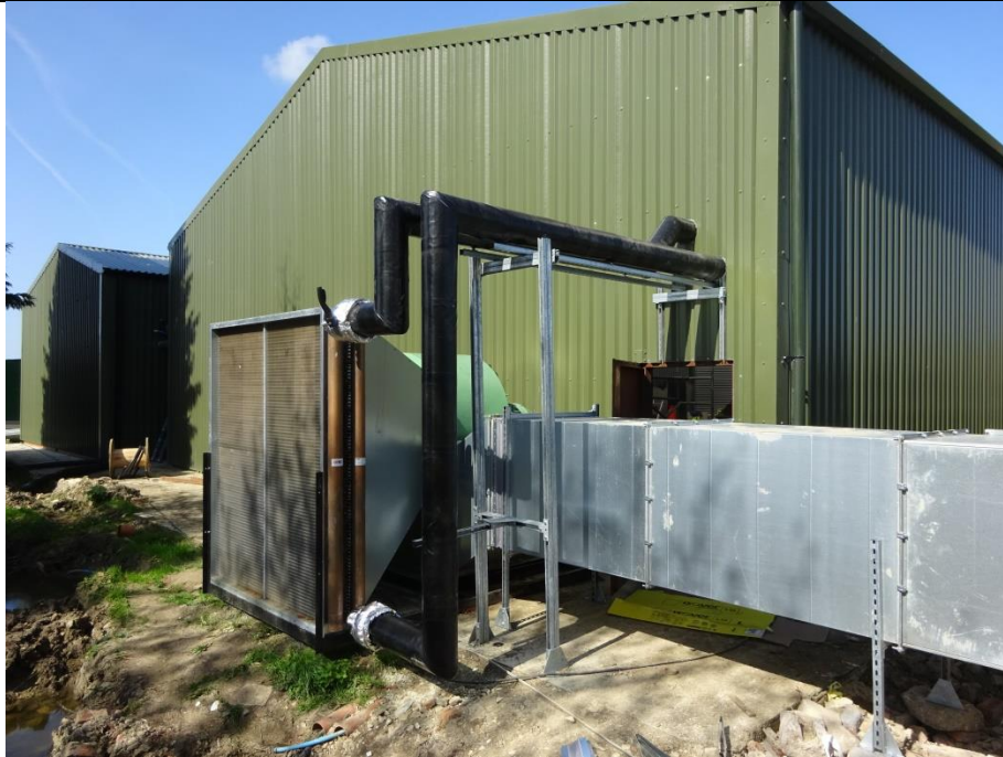
Dryer Fan and Heat Exchanger Behind Fully Enclosed Boiler house
