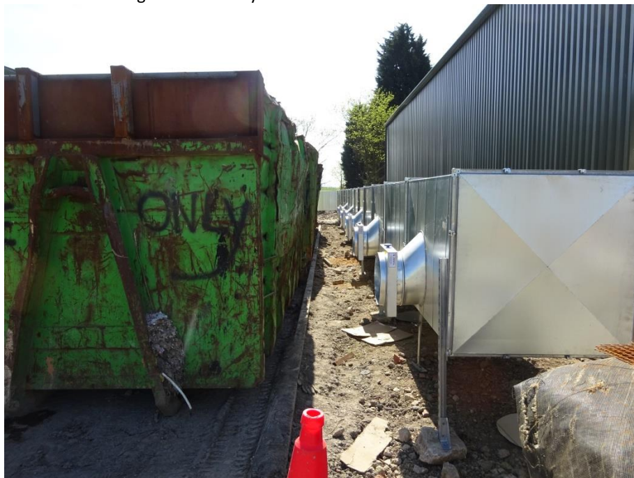
Ducting for Air Pipework into Hook Bins (Note: Hook bins not fitted at time of visit)
