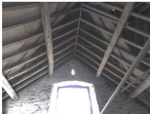
Fig. 24 Cobwebbed extended gable
