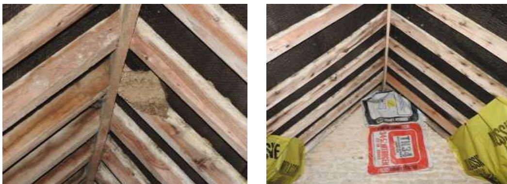
Figs. 12 & 13 Cobwebbed gable and ridge
