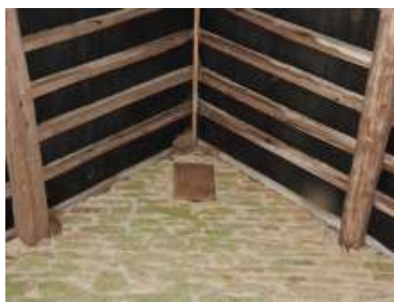
Fig. 11 Cobwebbed gable and ridge
