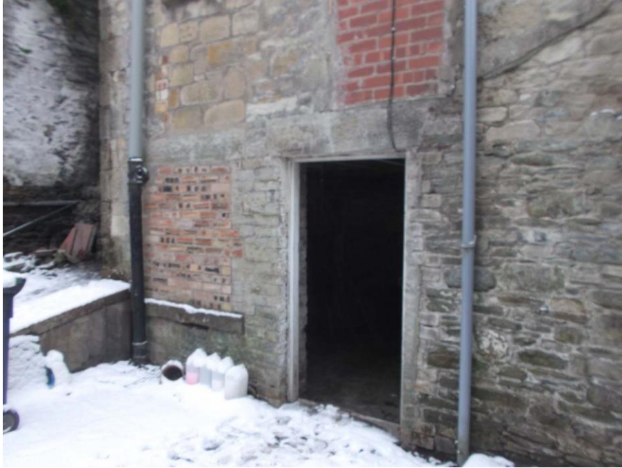
Photograph 3 – view of northeast elevation and door to basement (blocked openings visible)
