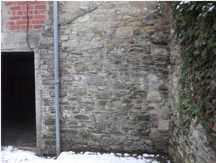
Photograph 4 – view of northeast elevation and door to basement (blocked openings visible)
