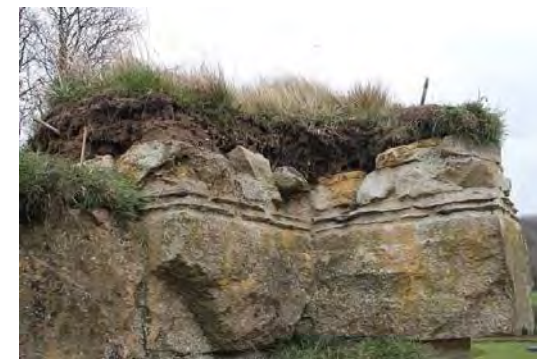
Example of soft capping applied to top of existing stone walls at Hailes Abbey, Gloucestershire Source: English Heritage
