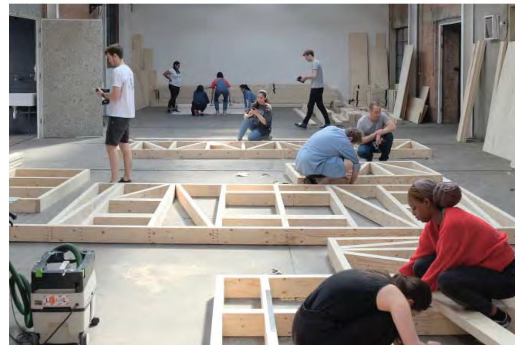
Construction of prefabricated timber wall panels, Maich Swift Architects, Potemkin Theatre self-build, London
