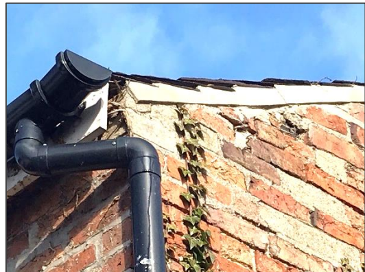
Photo 6: Gaps at gable end.
