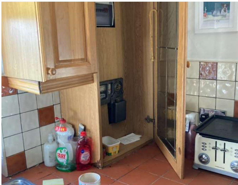
Location of the electric metre in The Annex
