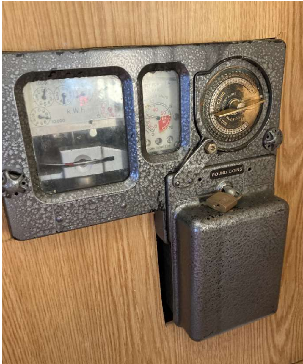
The Annex is served by a separate coin operated electricity metre
