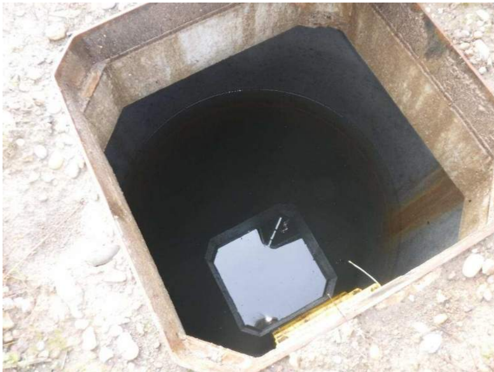
Plate 2: Borehole soakaway on 8 th October 2020.
