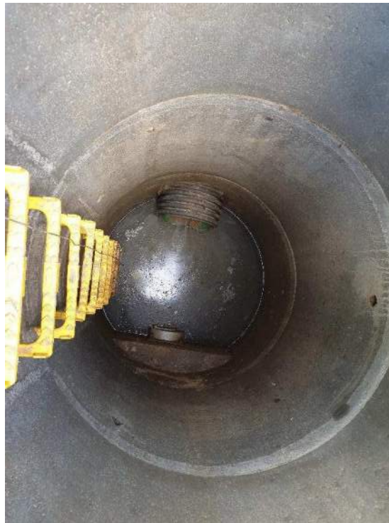
Plate 3: Hydrobrake (flow throttle valve) chamber on 29 th September 2020.
