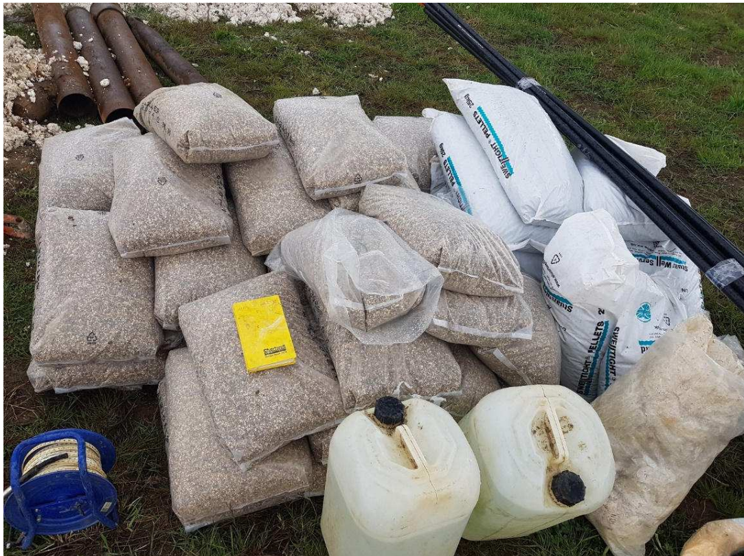
Plate 4: Backfilling materials consisting of granular 2 to 4mm diameter medium (gravel) and bentonite pellets.
