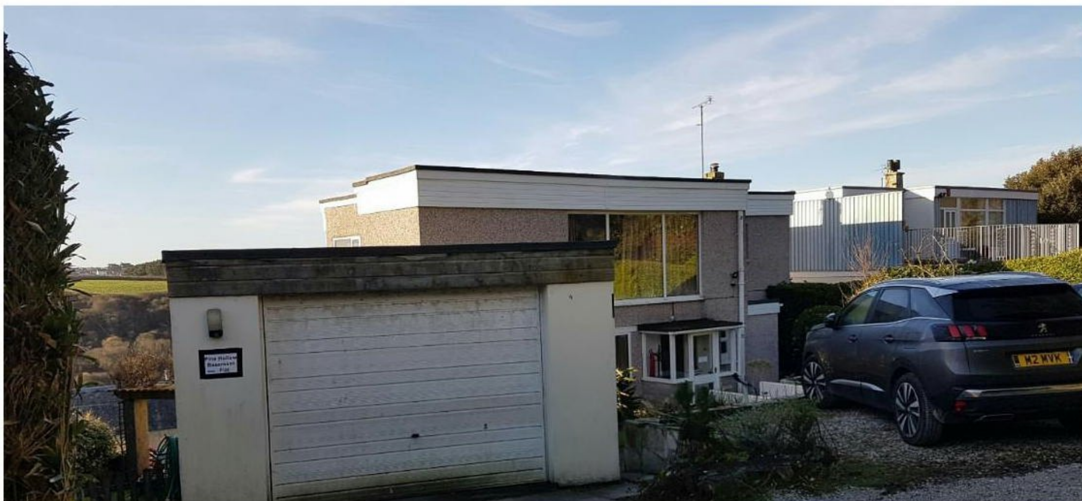
Existing View From The Private Drive (North) Showing unsightly and misaligned garage and weathered pebbledash
