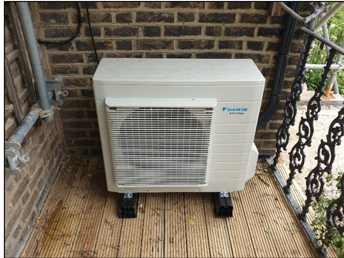
External Condenser Unit
