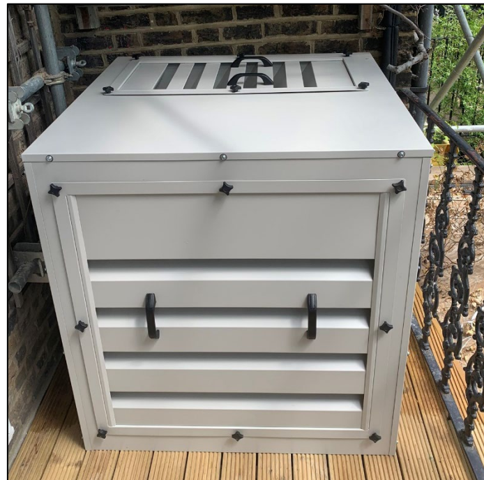
Condenser inside an Acoustic Louvre Enclosure
