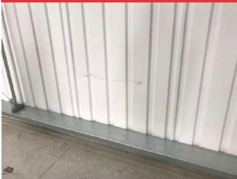
23 Damage to cladding.
