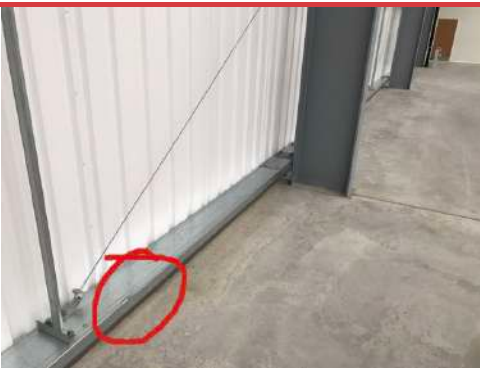
19 Dent in cladding rail.
