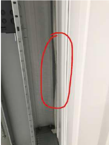
22 Dent in cladding.
