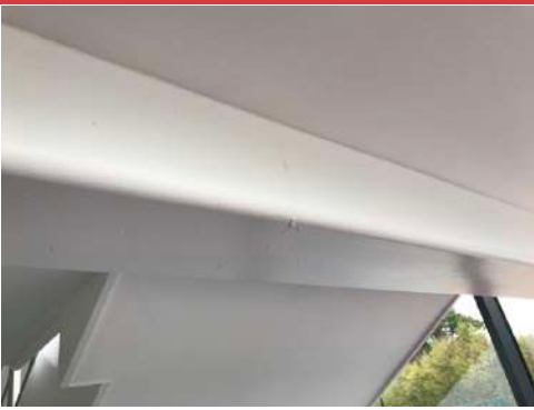
5 Paint splodge under stairs.
