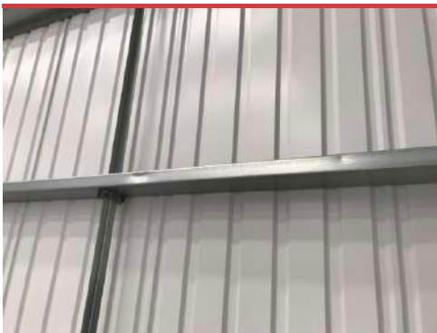
24 Dents in cladding.
