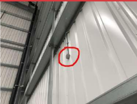
27 Penetration to have mastic.
