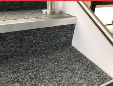
8 General note - Paint on stair carpet.
