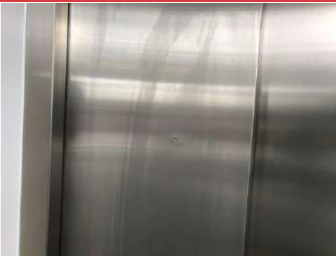
6 Dent in lift door.
