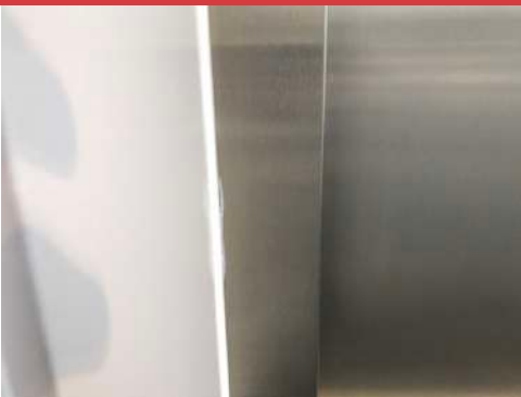
7 Over paint on lift trim.
