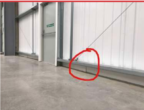
20 Gap in flashing.
