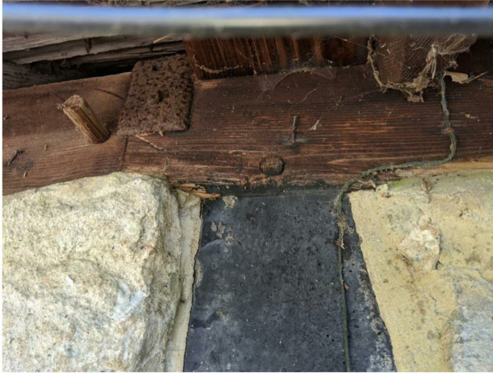
Figure 26: Wall plate joint where original/early timber pegs exist. The later metal bracket was added later, likely as a reinforcement to remediate structural issues.
