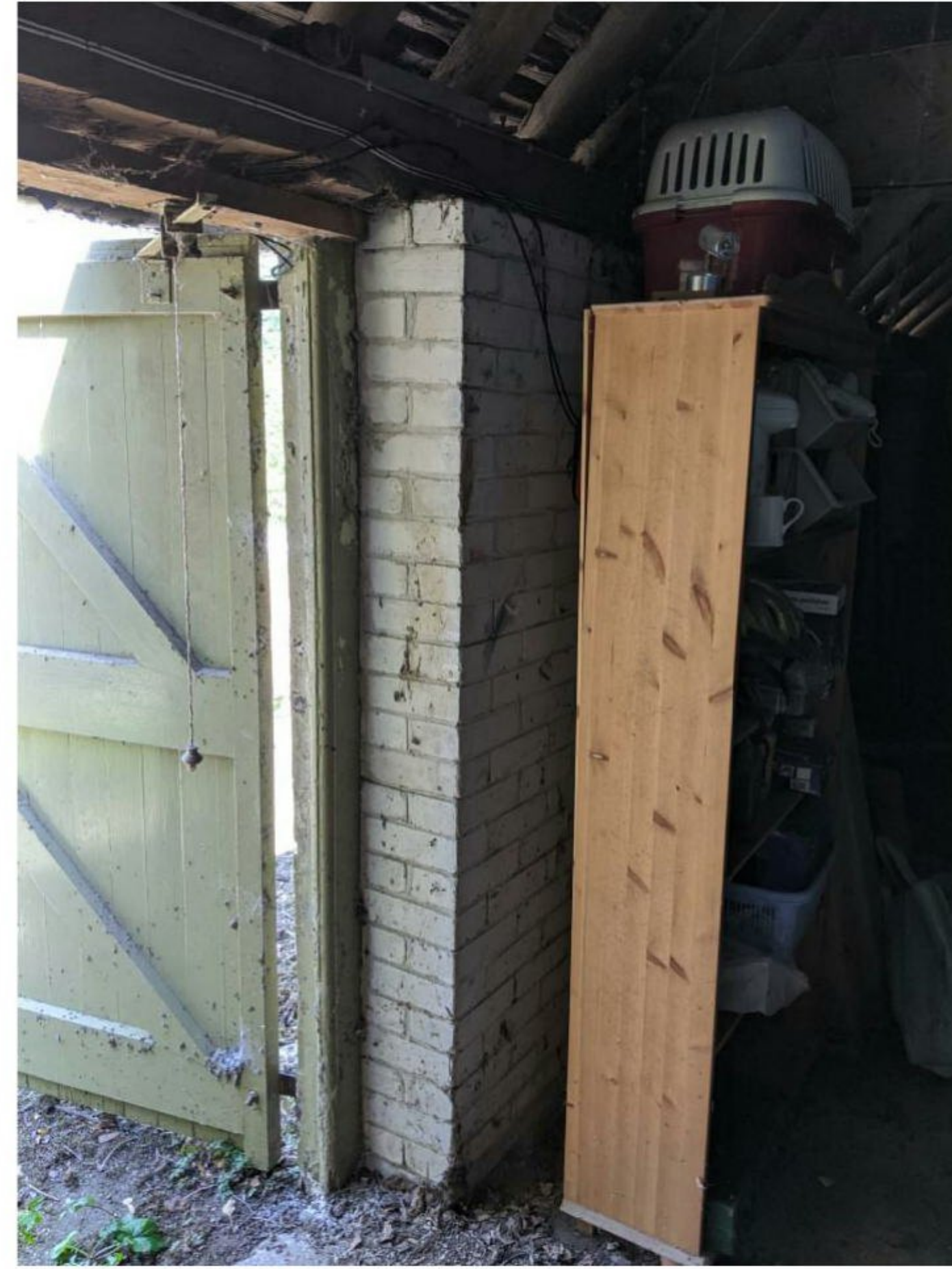
Figure 29: One of the north elevation openings showing the later white brick lining.
