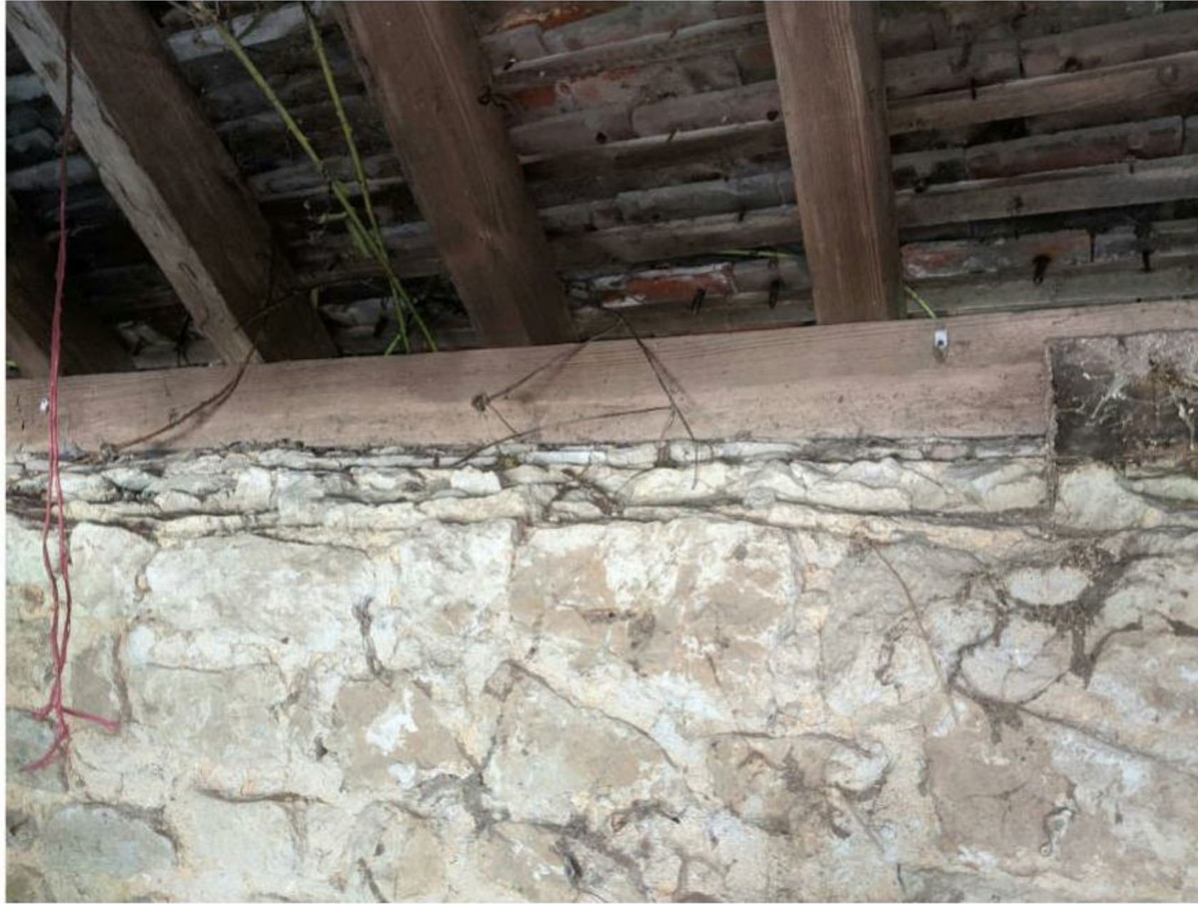
Figure 24: Timber wall plate and rafters directly placed above the rubble wall. The rafters and sections of wall plate do not have the patina of age for a 18 th century building. The timbers appear to be from the same date and mostly pine. The roof structure appears to be a later replacement.
