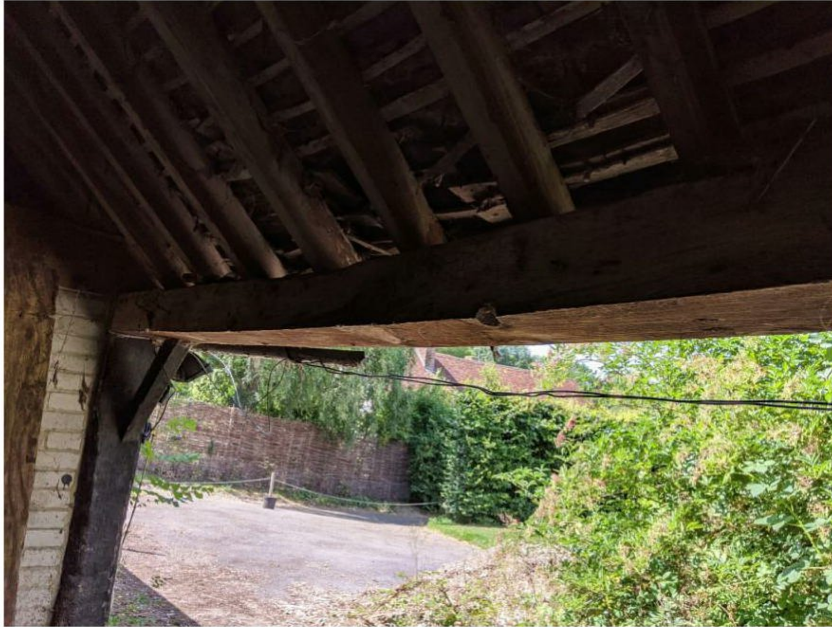
Figure 22: Larger opening in the north elevation of the barn. Lintel is sagging in the middle. Beams appear early/original and have a small brace on each side. New white brick lining on the inside.
