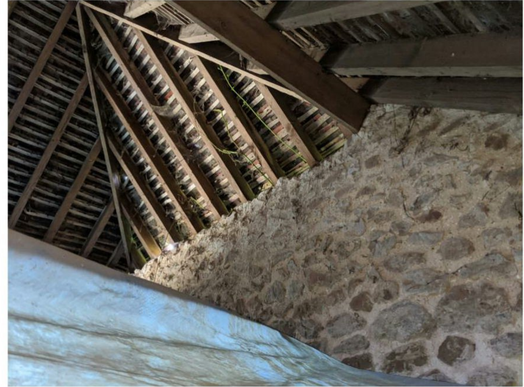
Figure 25: Internal view of the jerkinhead roof at the east elevation. Rafters, purlins, battens and roof tiles are visible.
