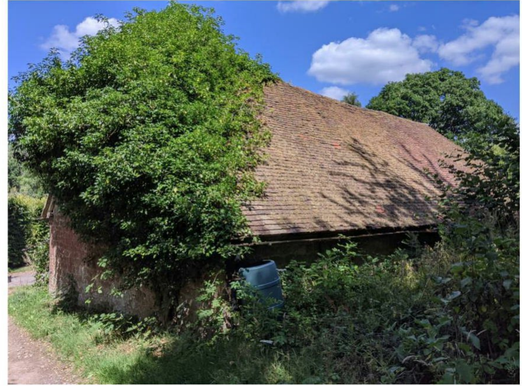
Figure 15: South 'rear' elevation of the barn. The land slopes up on this side.
