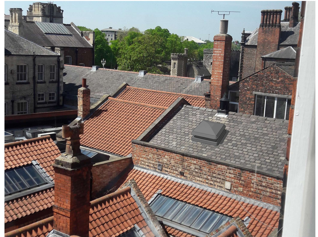
Photograph from first floor rear window of the application site, showing proposed cowl.
