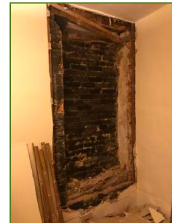
Original blocked window found in south-west elevation of the original core of the building (bedroom 3).
