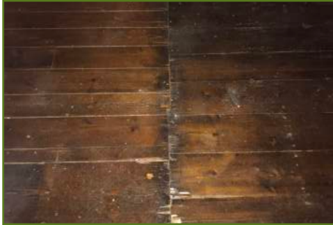
Join line of flooring in bedroom over the drawing room.
