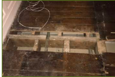
Trimmer and landing found after the removal of floorboards.
