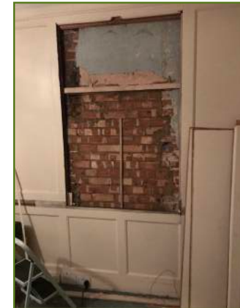
Modern brickwork and remnants of plaster found under panelling in bedroom over drawing room.
