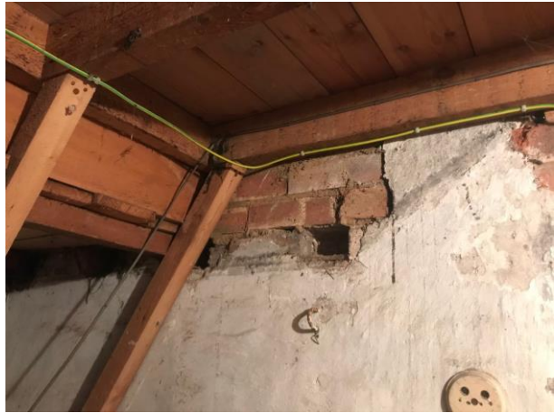
Photos from position 1 and 2 showing common brick upwards from height of original quarter landing. Evidence also of stairs being full width of stair well incorporating what is now the cupboard
