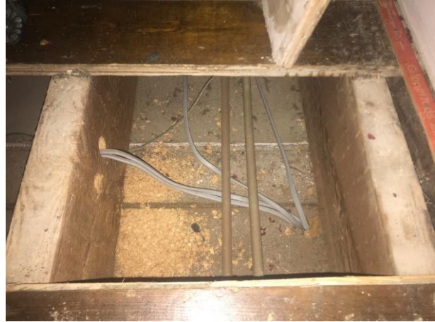
Photos from position 6 showing modern joists and floorboards forming landing to bedroom 5
