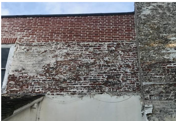
Above - evidence of bricked up window revealed through poorly toothed in brickwork
