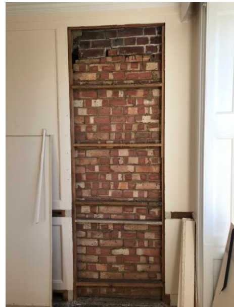
Photo from position 9 showing modern common brick of earlier doorway (highlighted orange on layout)
