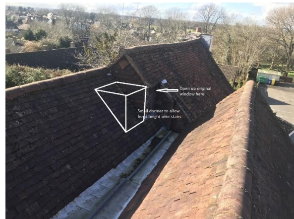
Indicative size and location of small dormer to allow head height over stairs to loft
