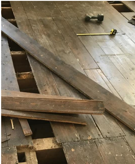
Photo from position 8 showing narrower boards in pale yellow section of bedroom 5 floor.
