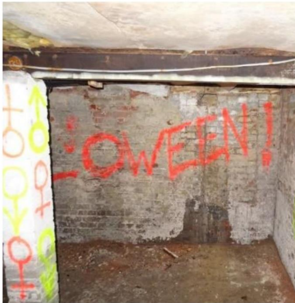
Showing view of NW wall of basement under drawing room (graffiti by others)
