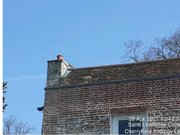
Figure 11: Further example of gaps between loose and or missing roof tile.
