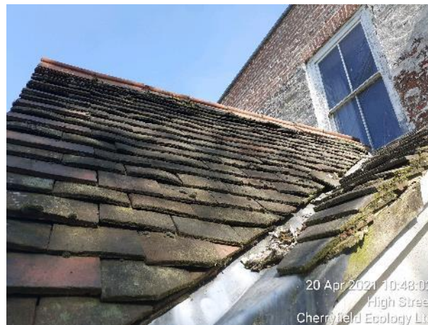
Figure 13: Further example of gaps between loose and or missing roof tile found on the roof of the front porch area.
