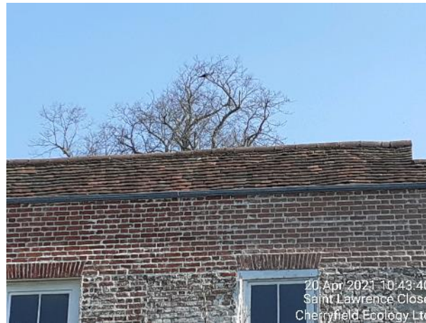
Figure 12: Further example of gaps between loose and or missing roof tile.
