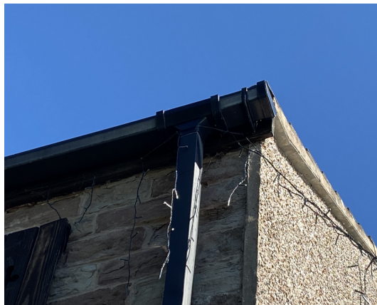
PHOTO 2 - House fascias soffit detail - no gaps
