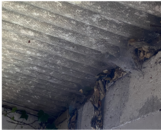
PHOTO 5 - Cobwebs internally within Store building
