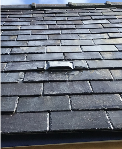
Ref: Bat 1 West facing 'Just Lead bat access slate' with 1F bitumen felt enclosure
