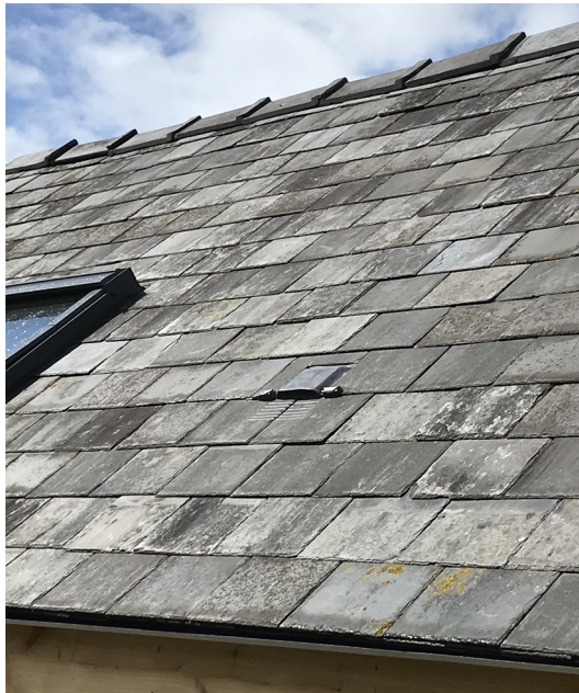
Ref: Bat 3 East facing 'Just Lead bat access slate' with 1F bitumen felt enclosure
