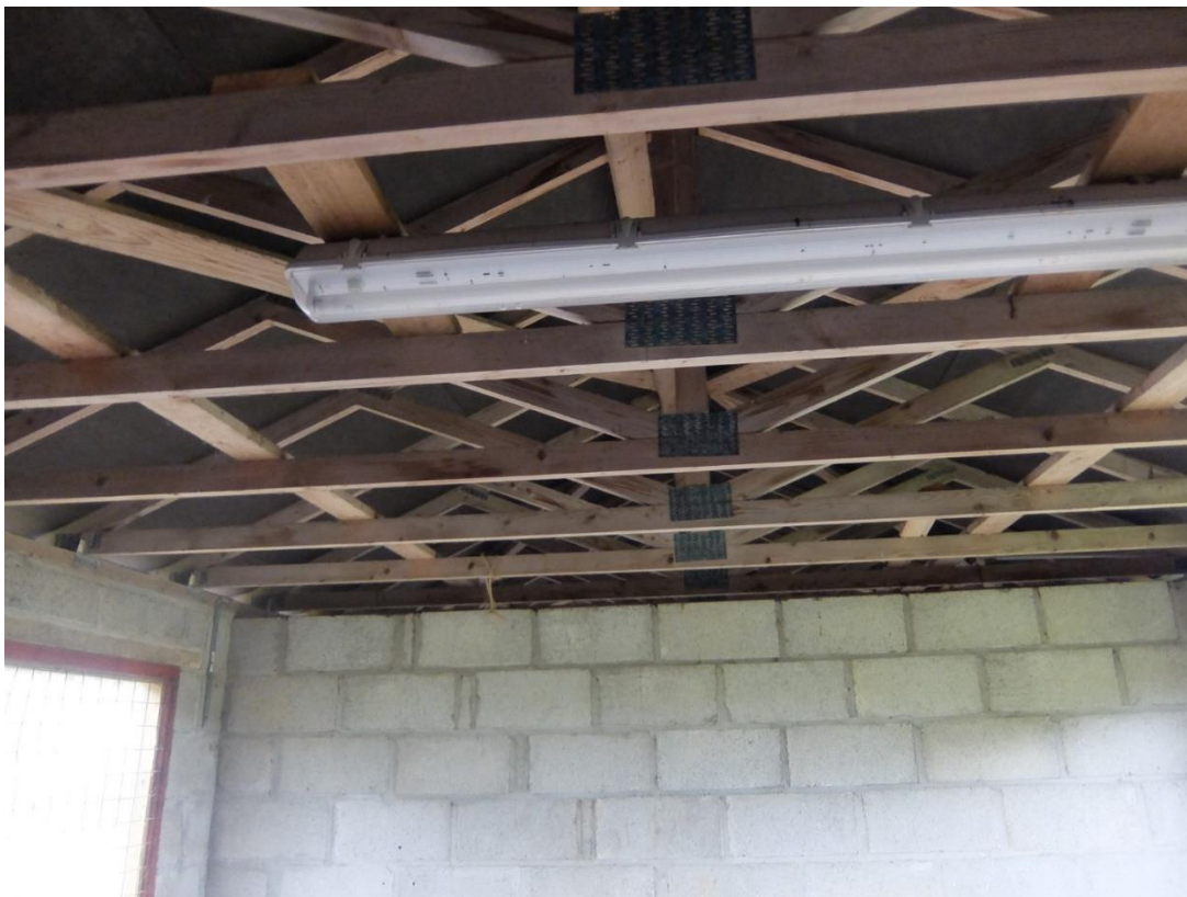
Roof structure showing trusses at close centres with lateral and diagonal wind bracing
