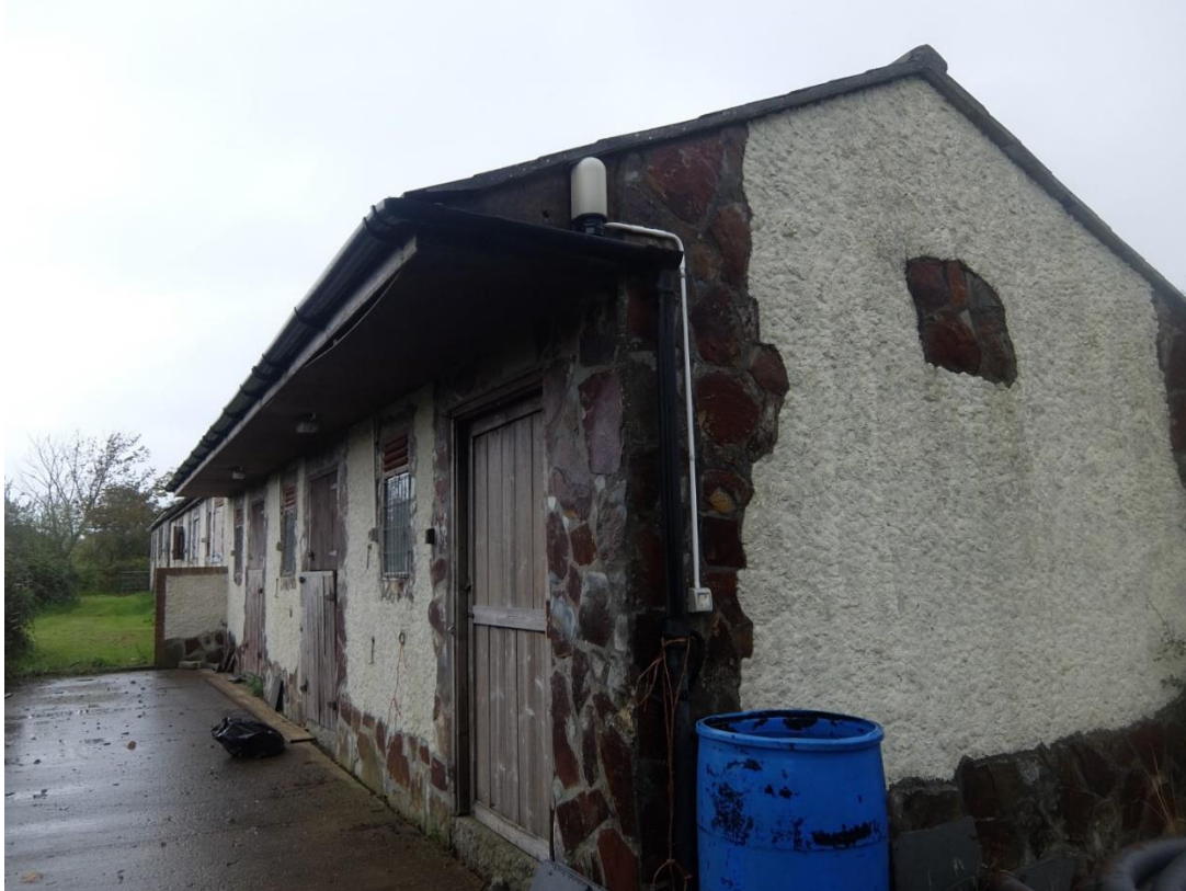
Front and left side elevations of whole building from attached storage bay side
