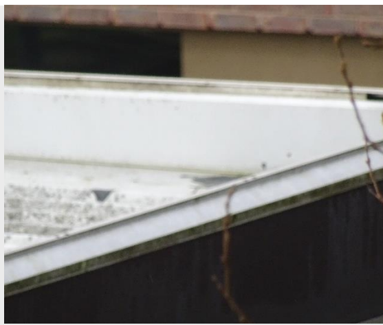
Photograph 3. Upstand of roof: photo taken from Top level- indicates there is no flashing material that bats can infiltrate.
