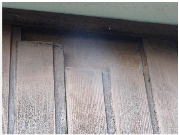
Photograph 8 may have limited potential for access on east flank wall as cladding has gaps
