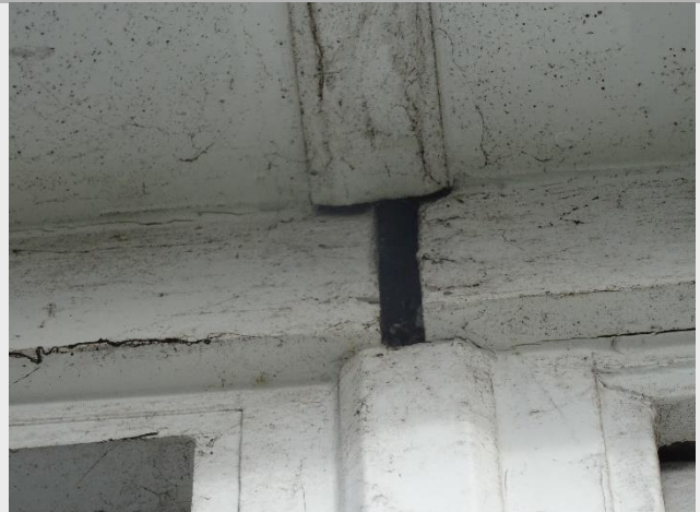
Photo 10. Hole in fascia marked by arrow at photo 9
